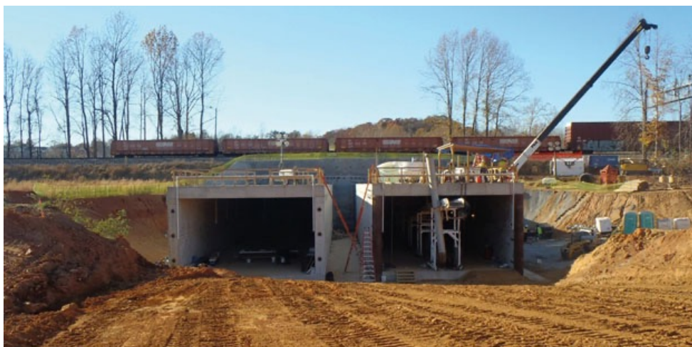
Figure 3-7 Example of jacked box tunneling method - Liberty University Tunnel, first jacked box tunnel in U.S.
