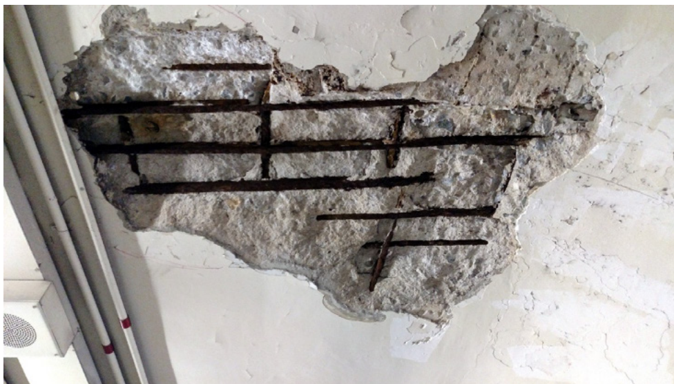
Figure 5-13 Example of spalling concrete from tunnel ceiling
