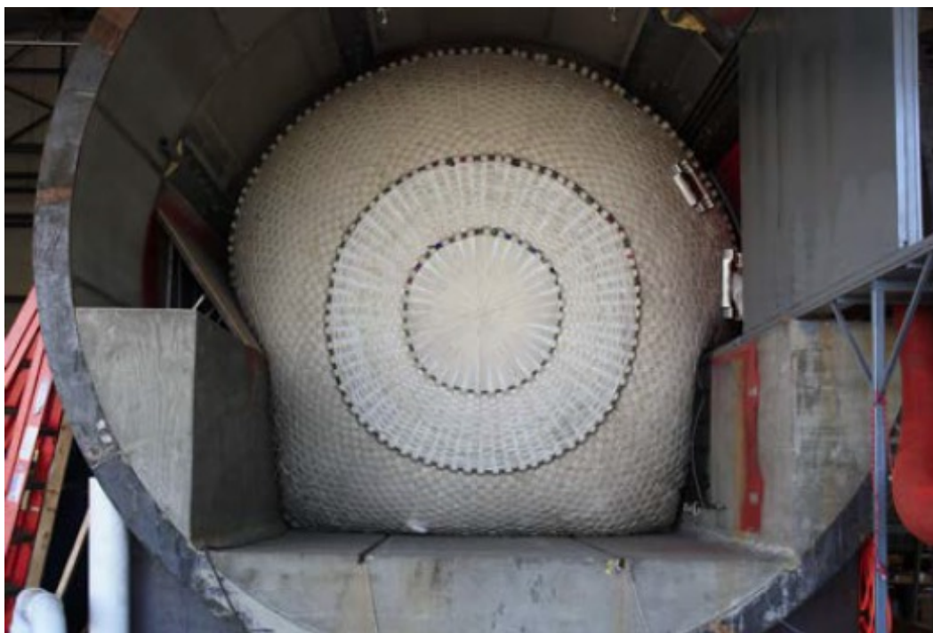
Figure 3-11 Photograph of the RTP (DHS 2014)
