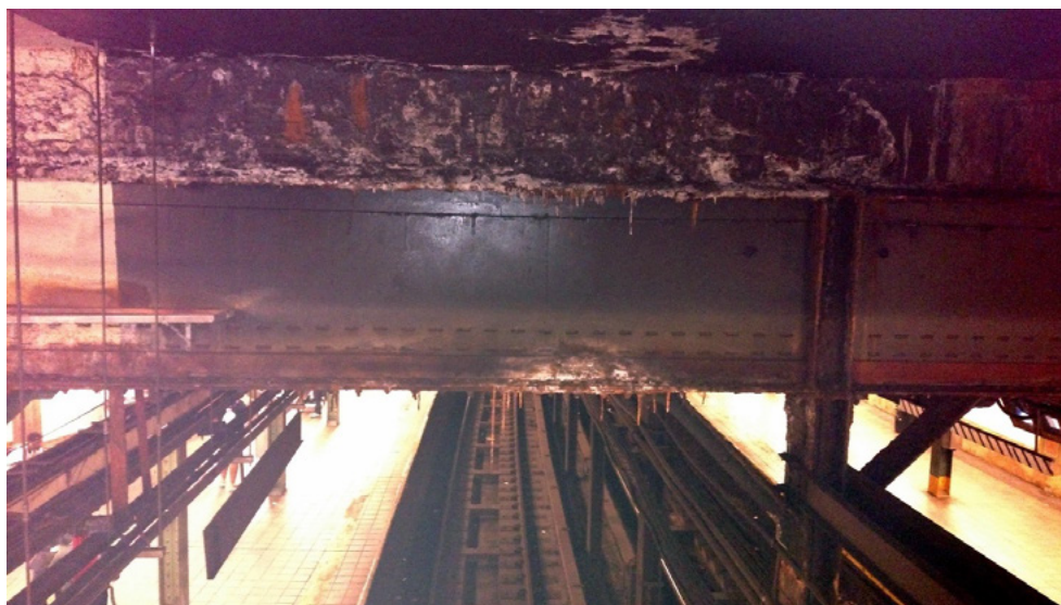
Figure 5-9 Example of leakage and corrosion on beam (view from station)
