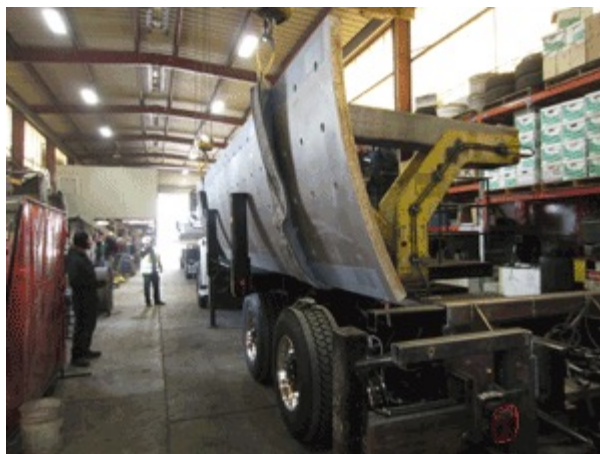
Figure 5-1 Custom-built plate-handling vehicle inside fabrication building carries steel plate used for reinforcement ( bart.gov )
