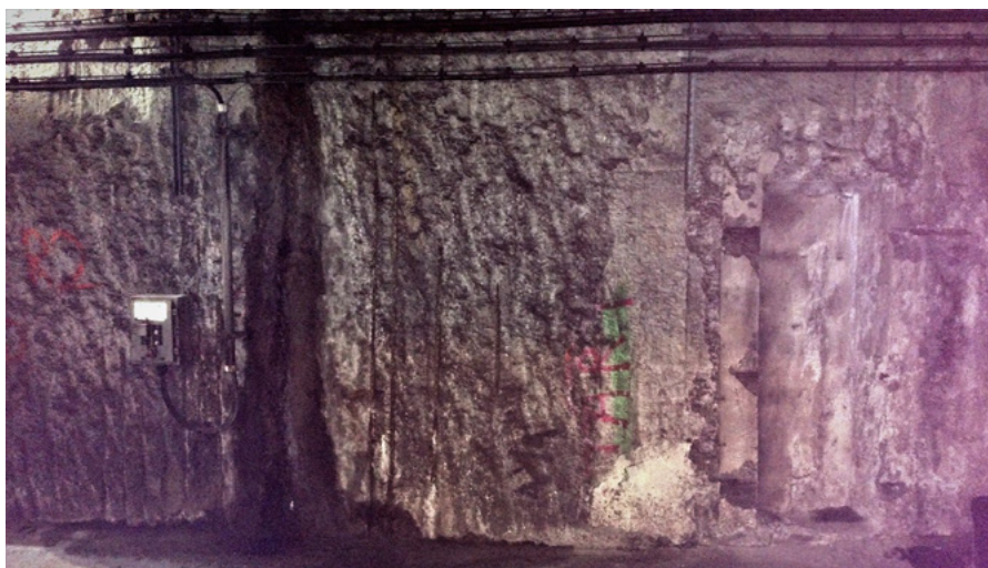
Figure 5-10 Leak on tunnel wall, deteriorated concrete, and exposed rebar
