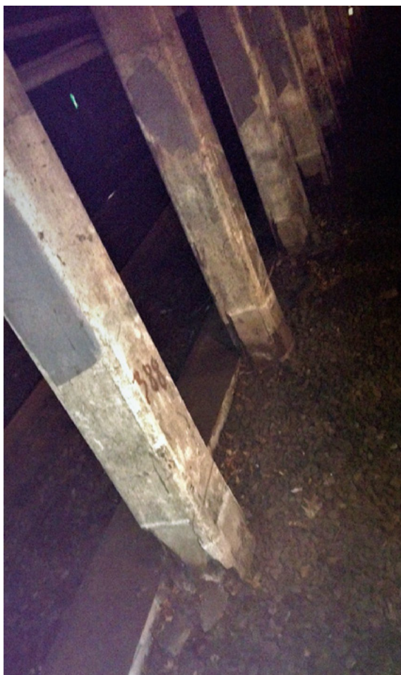
Figure 5-12 Deteriorated concrete columns
