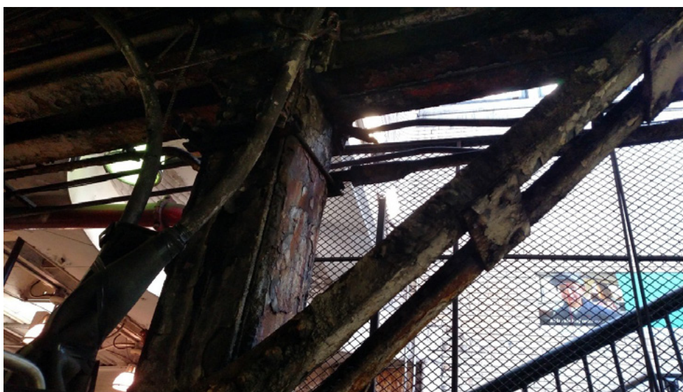
Figure 5-14 Example of deteriorated steel columns
