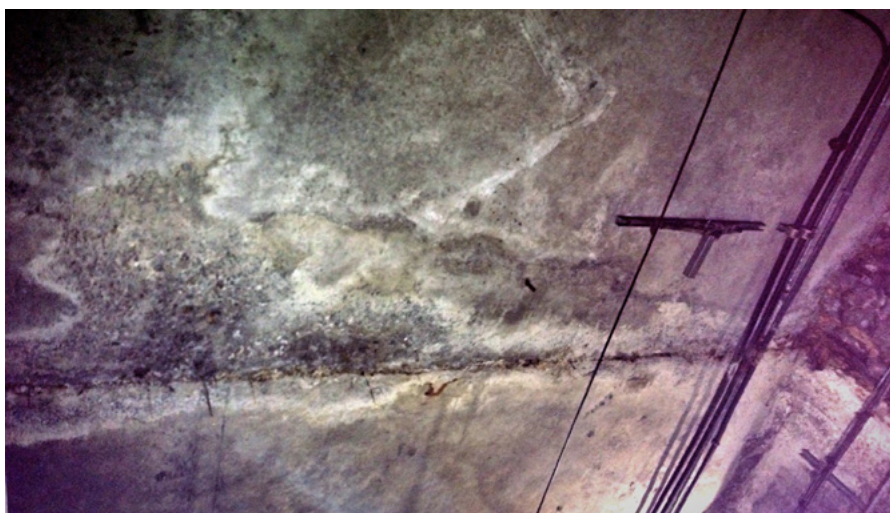
Figure 5-11 Leak on tunnel ceiling, efflorescence confirms salt in water
