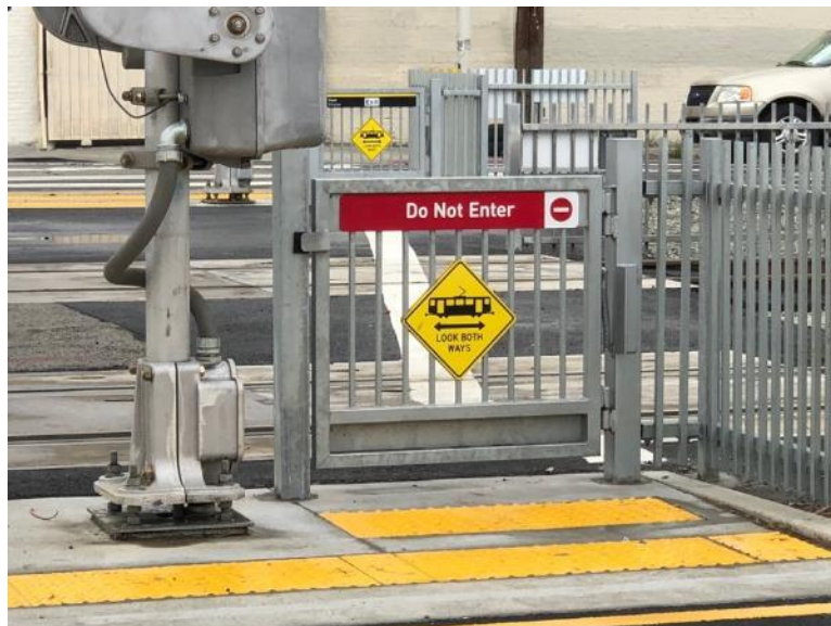
Figure 38: Pedestrian swing gates
