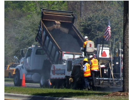
Using recycled asphalt pavement in new pavements saves money in road building and helps protect the environment.
