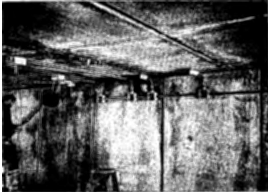
Figure 29. Soffit wiring with connections to anode and reference electrode.
