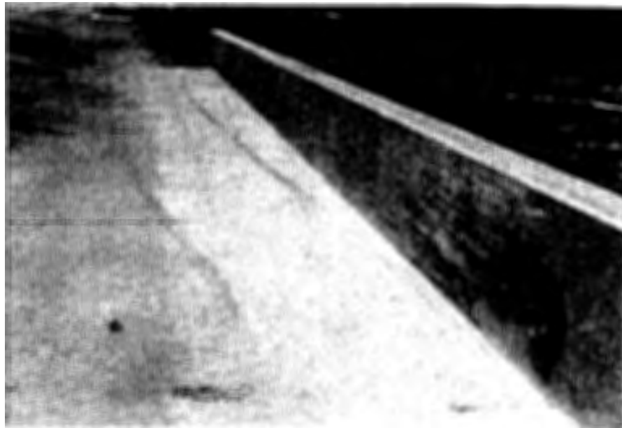
Figure 5. 32-in (813-mm) concrete parapet after test 7069-5.
