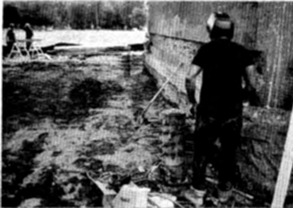
Figure 21. Welding shear studs onto micropile casing prior to incorporation into new reinforced concrete ground beam.
