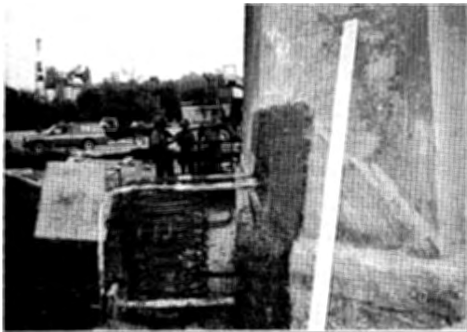
Figure 22. Reinforcement placed around micropile head prior to pouring of concrete ground beam.
