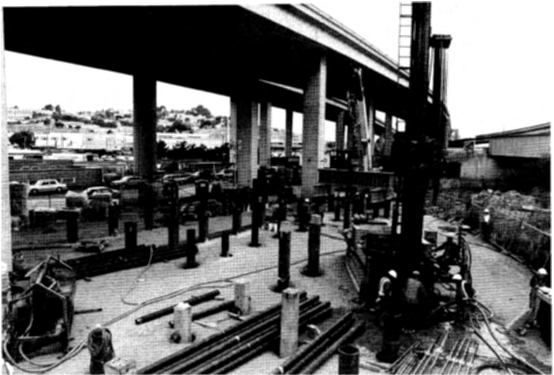
Figure 2. Long mast diesel-hydraulic track rig installing test micropiles. Reinforcement consists of both drill casing (bottom center) and bars (with centralizers, bottom right). Typical grout mixer/pump unit shown at bottom left.
