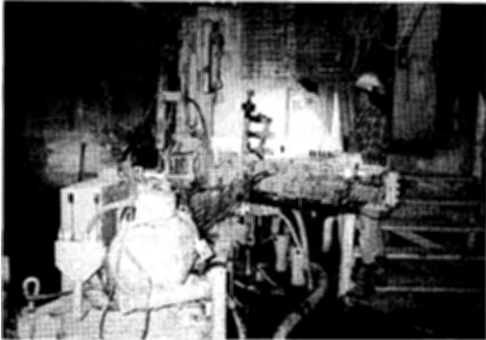
Figure 3. Short mast electro-hydraulic drilling rig operating in very restricted access and overhead conditions.
