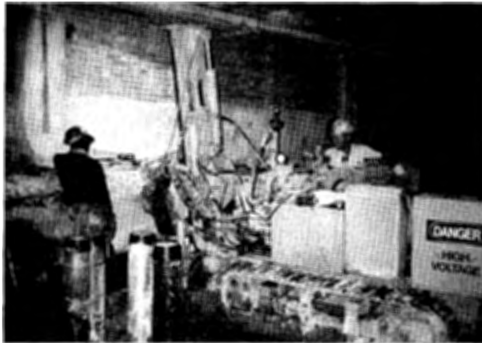
Figure 8. Electro-hydraulic track rig with short mast, used for micropiling in low-headroom conditions. [Note: Tracks withdraw inwards to permit rig movement through narrow openings.]
