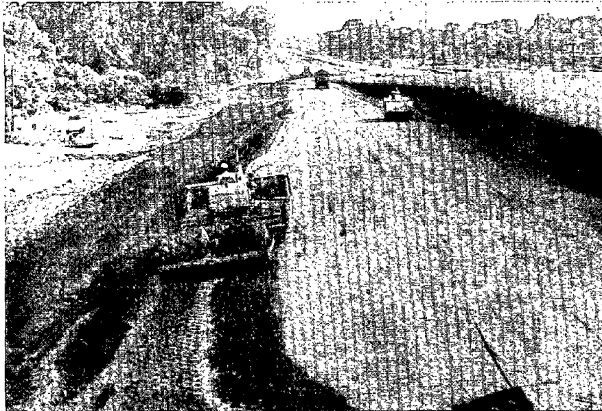
Figure 44. Compaction of fly ash embankment with vibratory roller and soil berm with sheepfoot roller.
