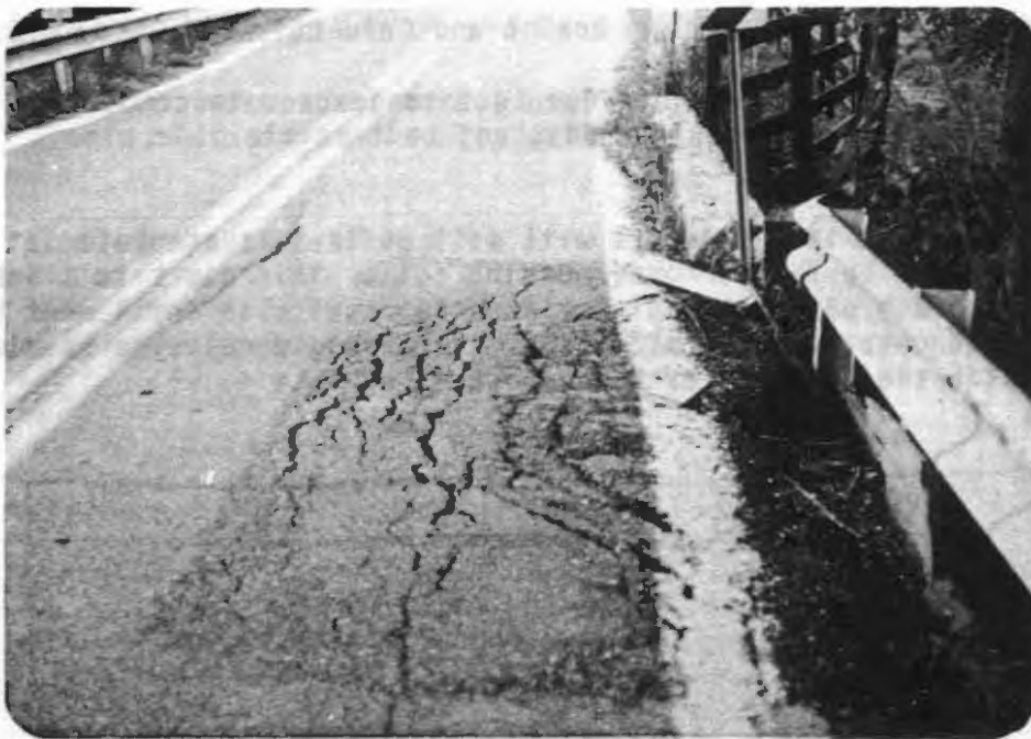
Exhibit 47. Pavement patches and pavement distress beside culvert. Distress is being caused by embankment spilling over wingwall.
