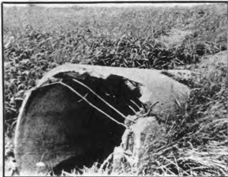
Exhibit 57. Impact damage to end of concrete pipe.
