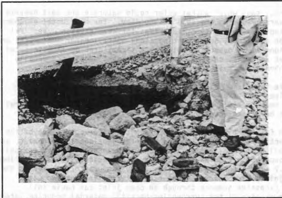
Exhibit 68. Surface hole above open joint.
