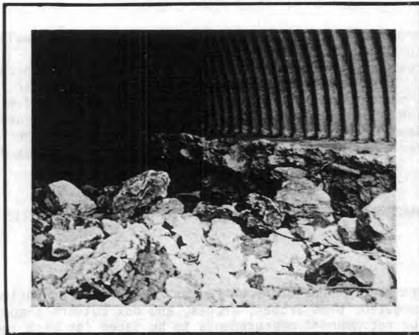
Exhibit 78. Erosion of invert undermining footing of arch.
