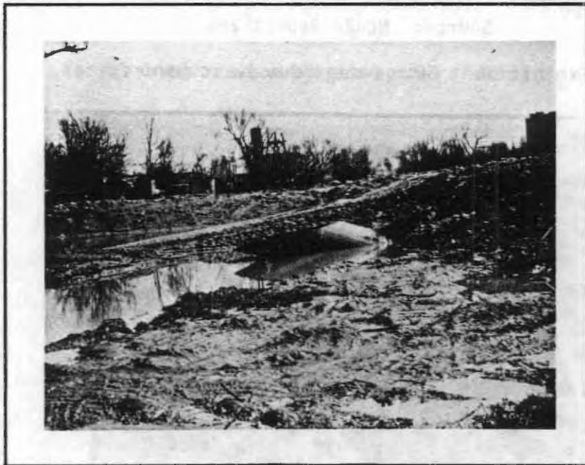
Exhibit 55. Mitered end of culvert turned up due to bouyant forces.
