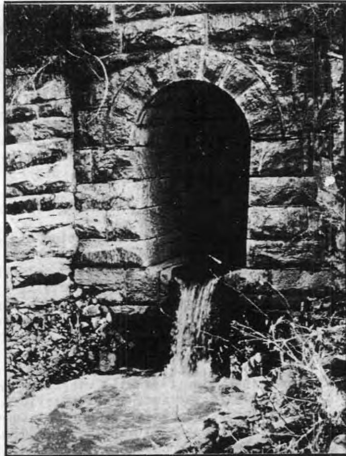
Exhibit 60. Scour at outlet of masonry culvert.
