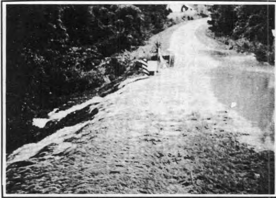
Exhibit 63. Culvert failure due to overtopping.
