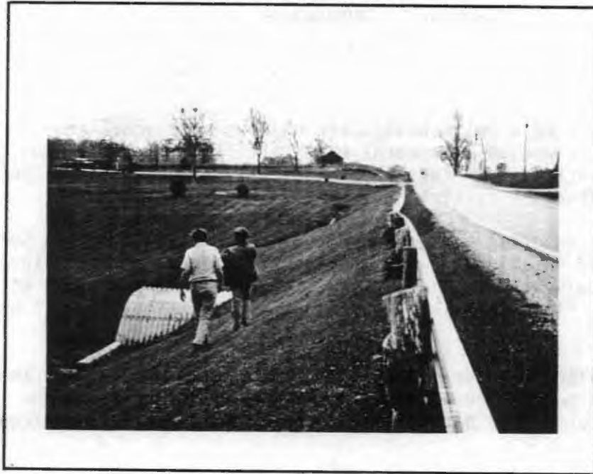
Exhibit 44. A dip in the guardrail or approach roadway may be due to excessive deflection in culvert.
