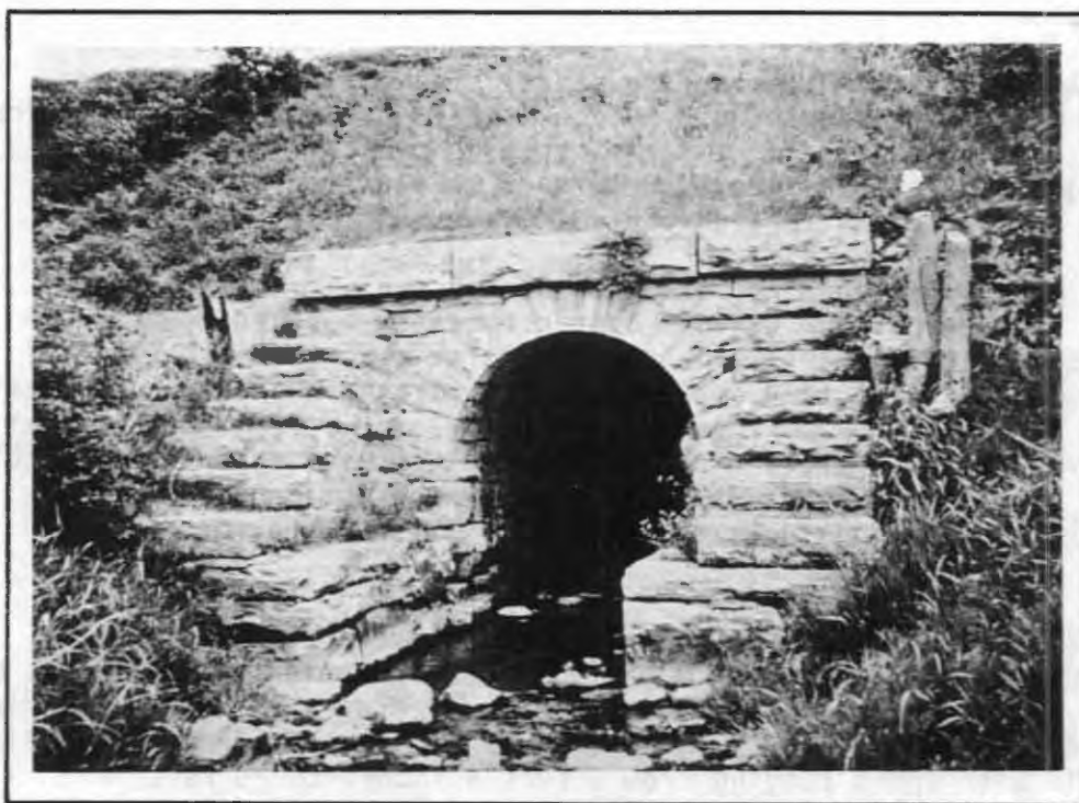
Exhibit 13. Masonry arch culvert. In some areas masonry arches and masonry box culverts are common. With good foundations these culverts have long service lives.
