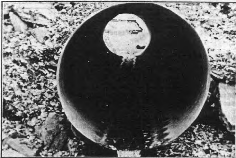
Exhibit 53. Voids around outside of pipe indicate possible piping. Shape distortion has occurred.
