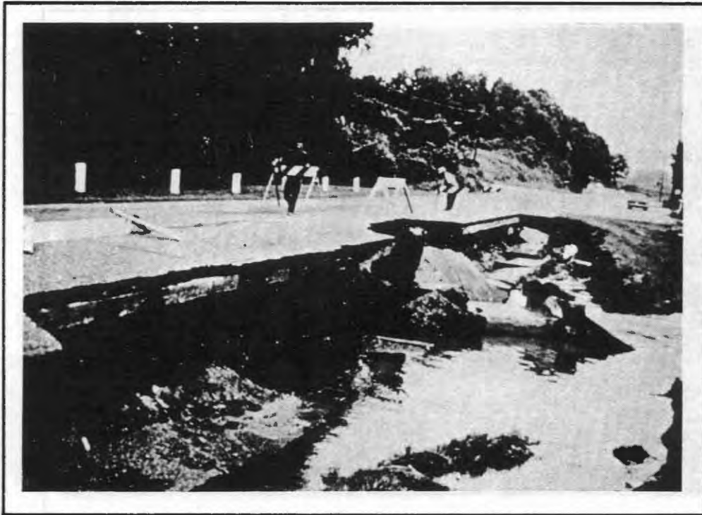
Exhibit 15. Roadway overtopping due to culverts with inadequate capacity may result in extensive damage to the roadway and the embankment.
