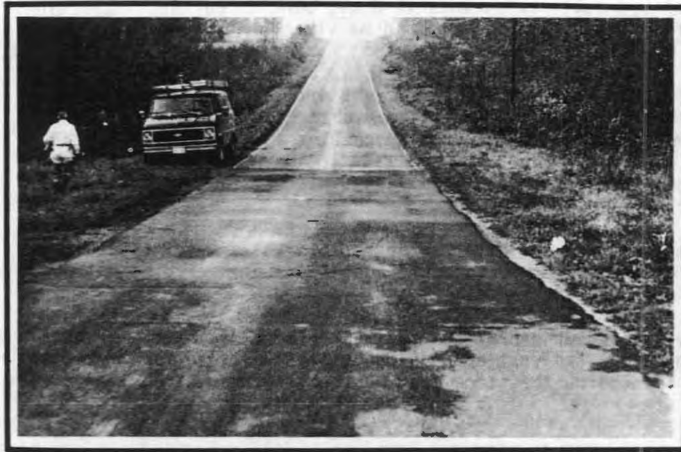
Extensive roadway patching due to settlement of the embankment.
