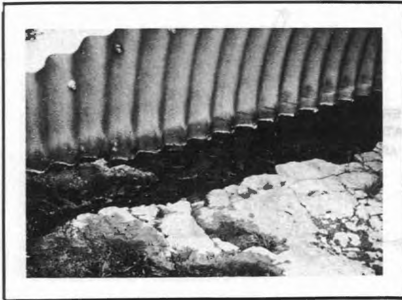
Exhibit 79. Erosion damage to concrete invert.
