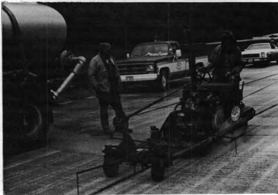
Figure 7. Concut diamond saw. This self-propelled machine was easy to operate, easy to keep in alignment, and made a very uniform recess. The truck on the left supplied the water to the saw via a hose.
