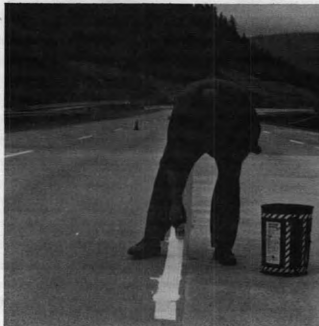
Figure 14. Workman sprinkling a topical application of glass beads over a completed section of Concrete 1064. Cure time on the epoxy is temperature-sensitive which means more traffic disruption on cool days.
