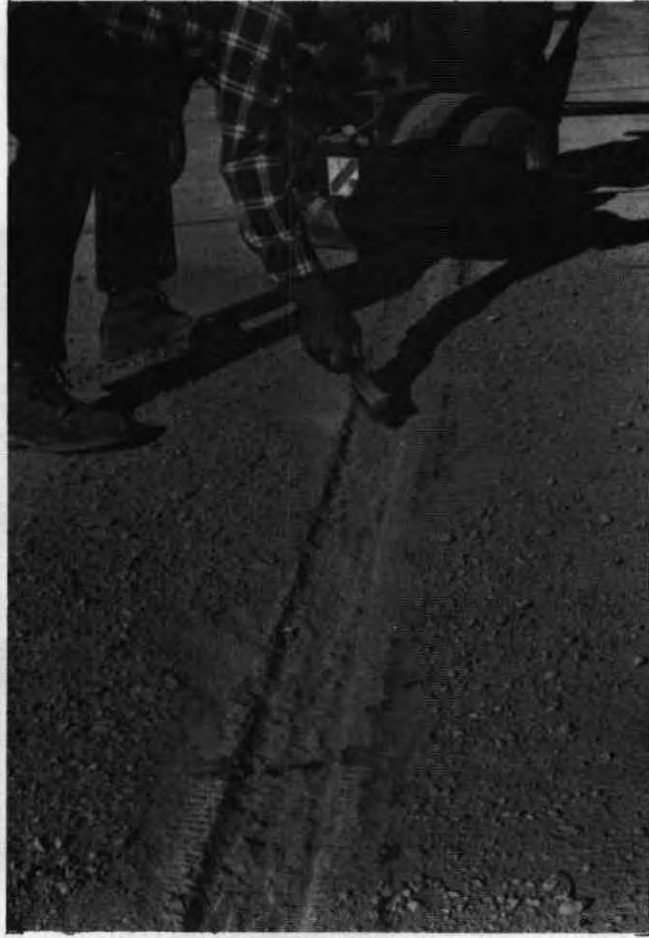
Figure 6. Recess formed by Tennant grinder. Note the uneven edges and variable cutting depth. A test cut in the asphalt shoulder had the same results.
