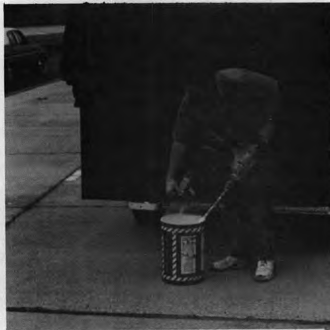
Figure 12. Mixing of Concrecive 1064 components and glass beads using a drill with mixer attachment. A generator in the trailer provided the power for the drill.
