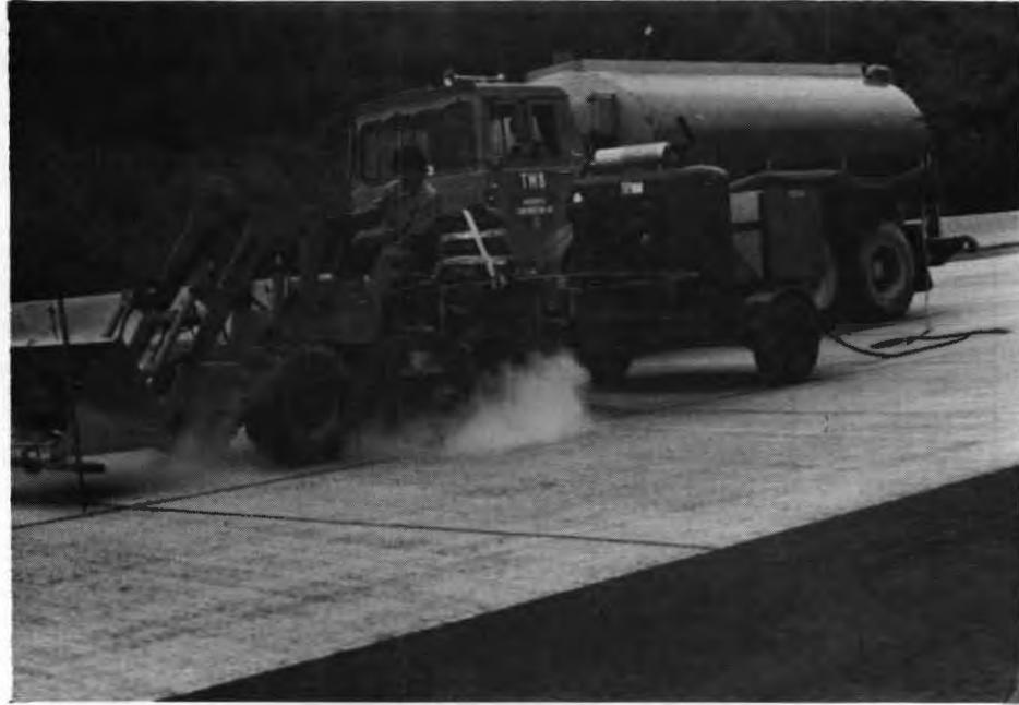
Figure 1. Flow Industries' water jet cutting system which includes a water truck, a trailer-mounted 60,000-psi intensifier powered by a diesel engine and an articulated front-end loader. The pressurized water is conveyed through a small pipe from the trailer to the cutting head.
