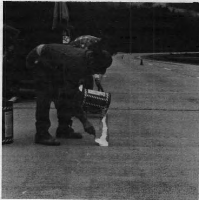
Figure 13. Workmen spreading Concrete 1064 material into a grooved pavement recess. The workman in foreground is using a trowel to spread the liquid epoxy. On a grade as shown (3%), it took extra care to distribute the epoxy and maintain a full-depth section throughout the recess.
