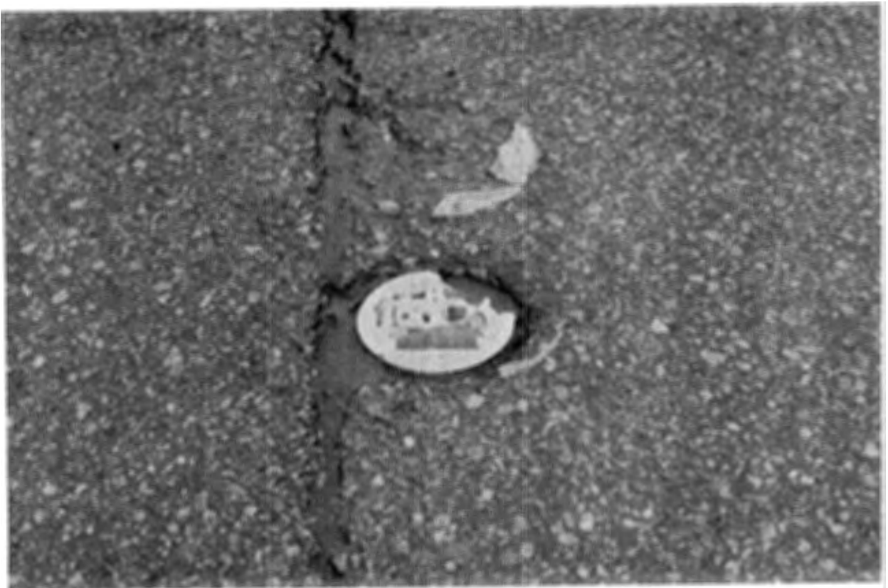
Figure 24. Damage to Kingray Marker by Snowplow.
