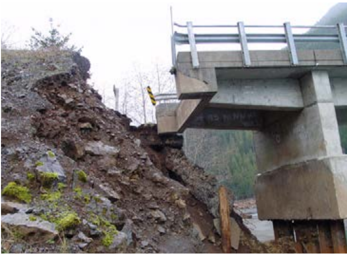
The eroded west approach of the Lake Cushman Bridge over the North Fork of the Skokomish River in Washington. The bridge is the primary access point to Olympic National Park.
