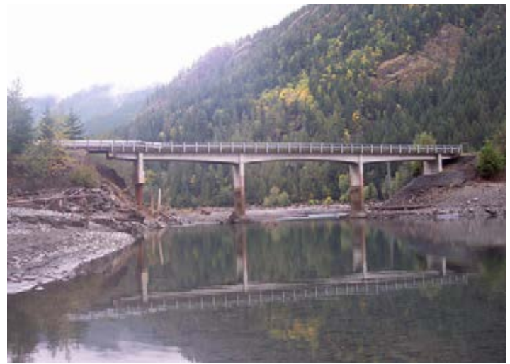
The new Lake Cushman Bridge stands ready for future river flows. To date, the bridge has not experienced a significant storm event since the repairs were completed.
