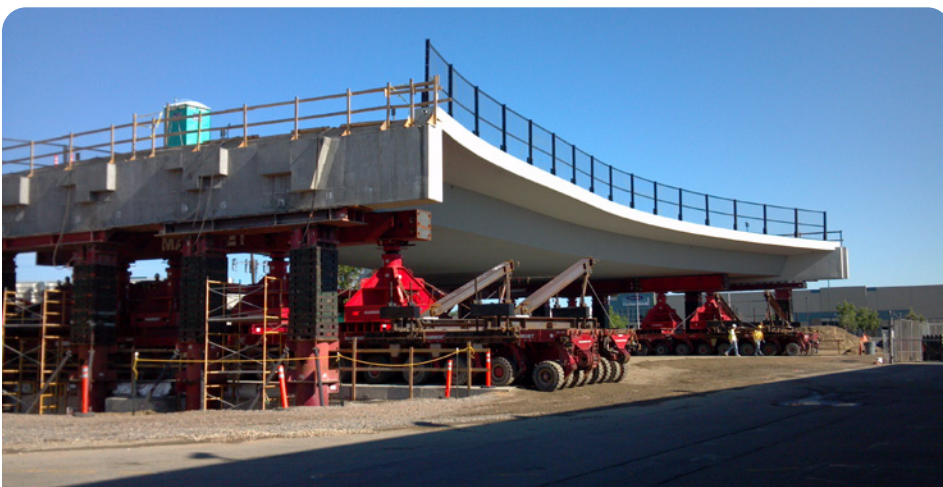
This bridge over I-70 and Pecos Street in Denver, CO, used prefabricated bridge techniques. Bridge elements were built near the site, lifted with hydraulic jacks, and moved into place using SPMTs. The bridge weighed 2,400 tons and took 50 hours to move 800 feet. Technologies like SPMTs enable the precise positioning of prefabricated bridge elements that can weigh thousands of tons.
