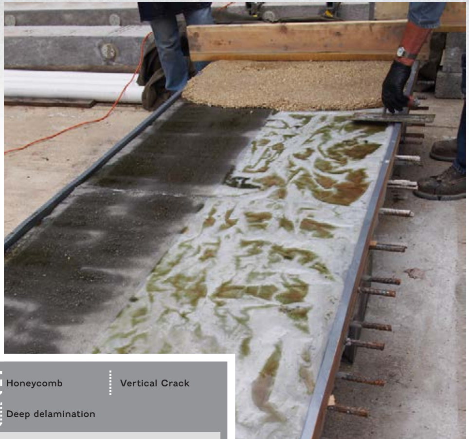
Silica fume-modified concrete overlays with a thickness of 1.5 inches (3.81 centimeters) were placed on S6. Source: FHWA.
