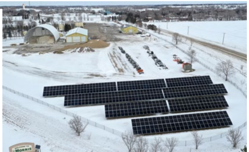
Solar Garden installation at a MnDOT operations and maintenance building in Morris, MN. © MnDOT.
