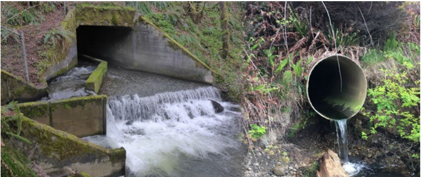
These two “perched” (outlet higher than the streambed) culverts may act as barriers to AOP, thereby disrupting long-stream connectivity and habitat functions of a river or stream. Fish trying to swim upstream would likely be unable to navigate the jump heights and the shallow water depths in the culverts.
