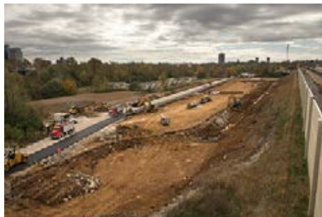
The NPEP mitigation area under construction. The noise wall can be seen on the right. The difference in elevation due to added fill can be seen in the center of the photograph.
