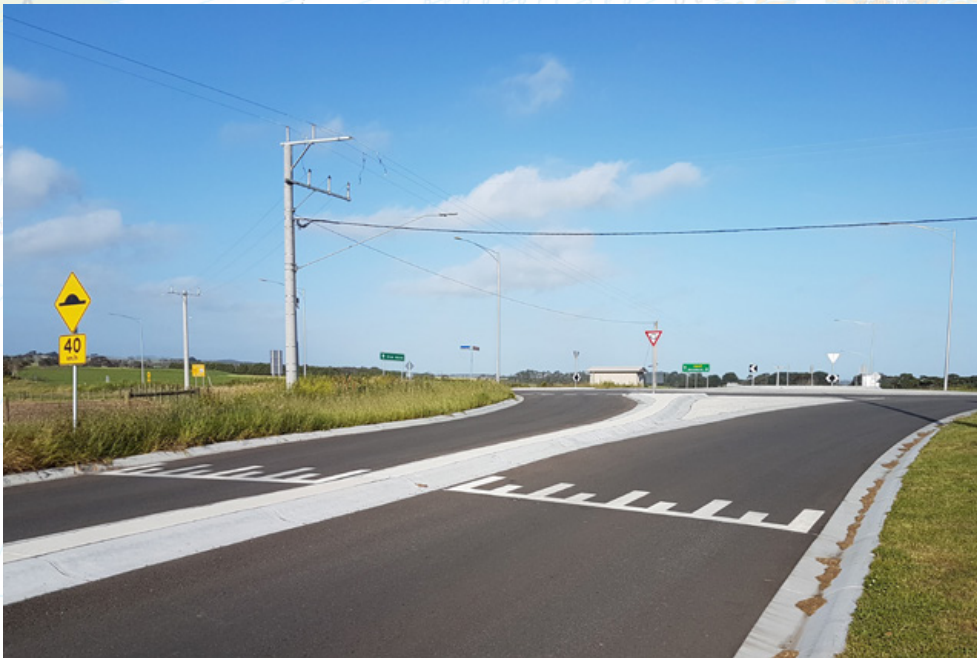
This high-speed roundabout in Victoria, Australia, uses a raised platform to manage speed.
