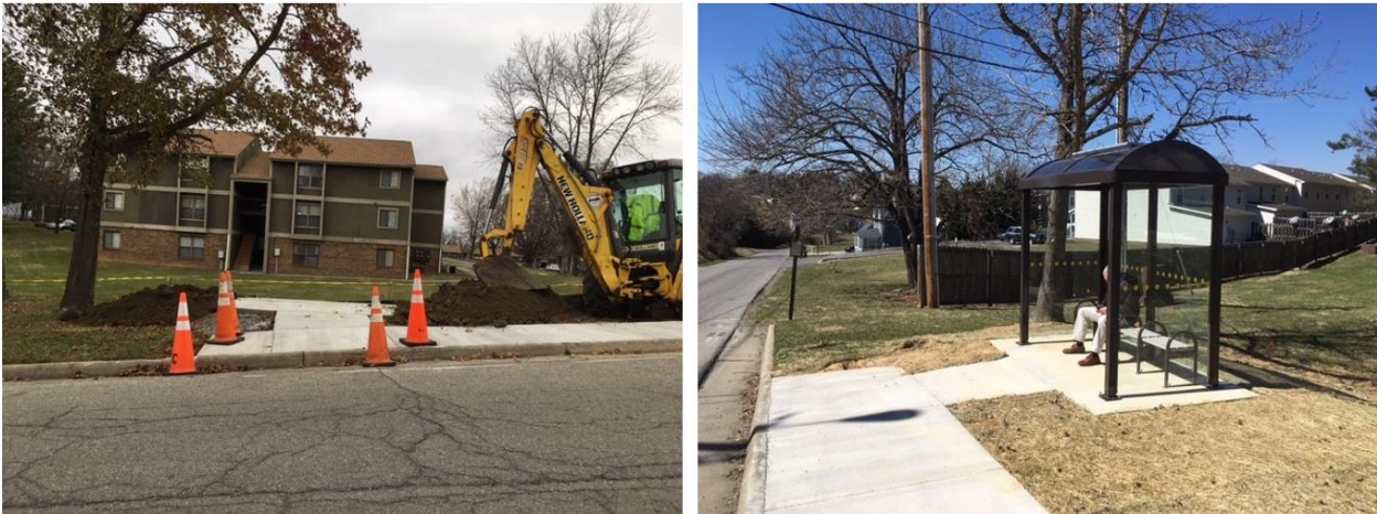
Figure 4. BT Stop 2101 During (left) and Shortly After (right) Construction. Images by Erik Olsen of BT.
