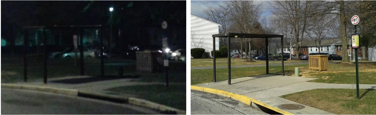
Figure 5. BT Stop 1414 Before Improvements at Night (left) and in the Daytime During Improvements (Electrical Connection Prepared) (right). Images by Erik Olsen of BT.
