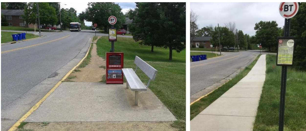
Figure 9. BT Stop 1328 Before (left) and After (right) Installation of Sidewalk. Images by Erik Olsen of BT.
