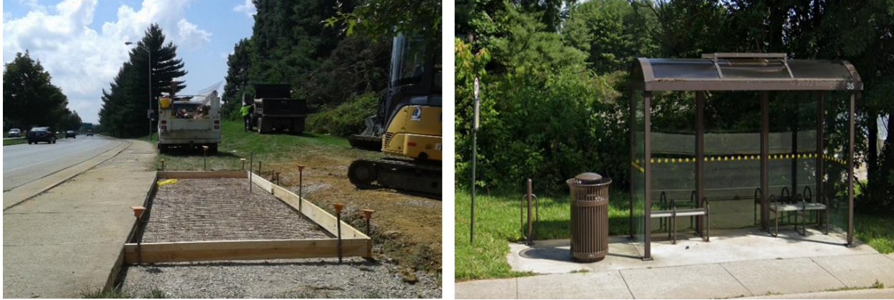
Figure 8. BT Stop 1200 During Improvements (left) (image by Erik Olsen of BT) and After Improvements (right) (image capture: June 2019 © 2023 Google).
