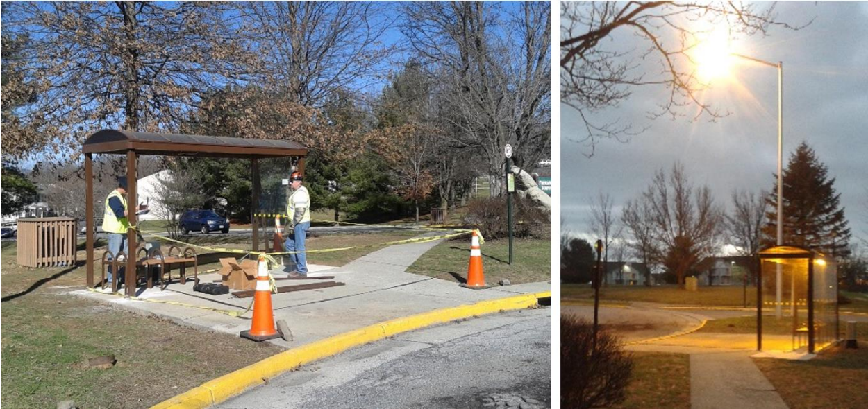
Figure 6. BT Stop 1414 During Installation of Reoriented Replacement Shelter With Bench (left) and After Construction Including New Street Lighting (right). Images by Erik Olsen of BT.
