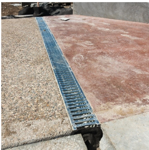
Figure 2.9 Trench drain. (Source: Mississippi Watershed Management Organization/Flickr)
