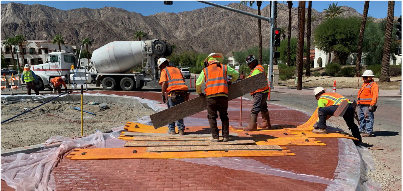
Figure 5. Photo. Another view of the intersection of Calle Tampico and Avenida Bermudas during improvement.
