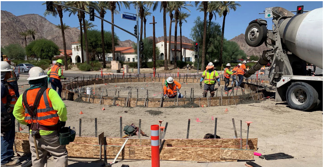
Figure 4. Photo. A view of the intersection of Calle Tampico and Avenida Bermudas during improvement.
