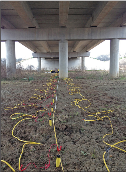
Electrode line array under Navasota River Relief Bridge at Brazos/Madison County Line, Texas.
