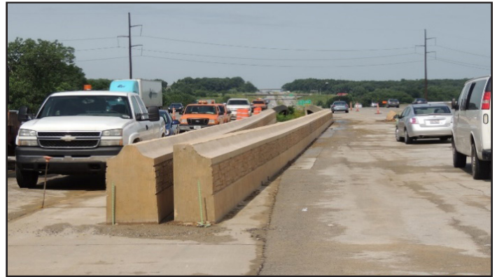
Figure 4. Implementation of the new concrete median barrier in Iowa. Note that the top of the barrier is more tapered than traditional designs. This new design reduces the probability of a vehicle occupant's head making contact with the barrier in the event of a crash.
