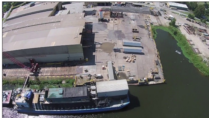
Figure 1. Construction of the first LNG bunker barge built in North America at Conrad Shipyard, Orange, TX, 2017
