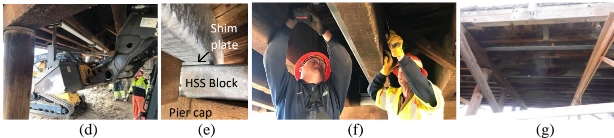
Fig. III.2. Repair with hollow structural sections (HSS): (a) schematic view; (b) HSS installation locations of F-22-V; (c) HSS installation locations of H-20-T; (d) lifting of HSS; (e) assembled HSS system; (f) drilling for connection; (g) completion
