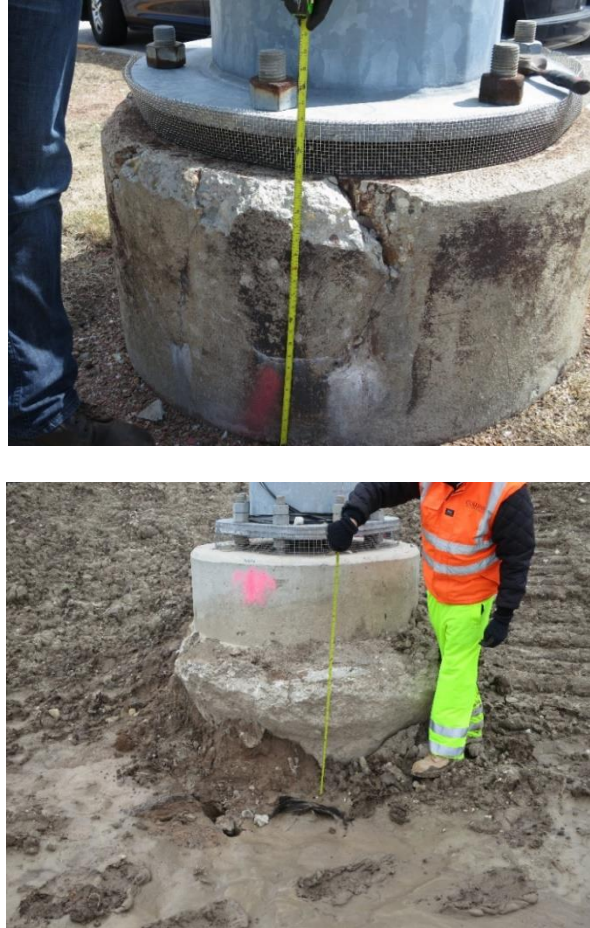
Figure 27. Photo. Spalled and exposed high mast lighting foundation ( WisDOT, 2017 ).
