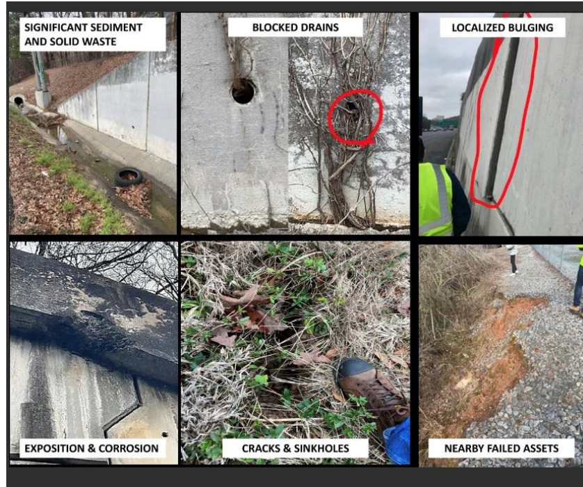
Figure 102. Photo. Examples of localized deterioration to cause failure.
