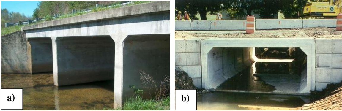
Figure 11. Photo. Examples of box culverts: a) triple barrel box culvert, b) single barrel box culvert. ( https://www.dot.state.oh.us ).
