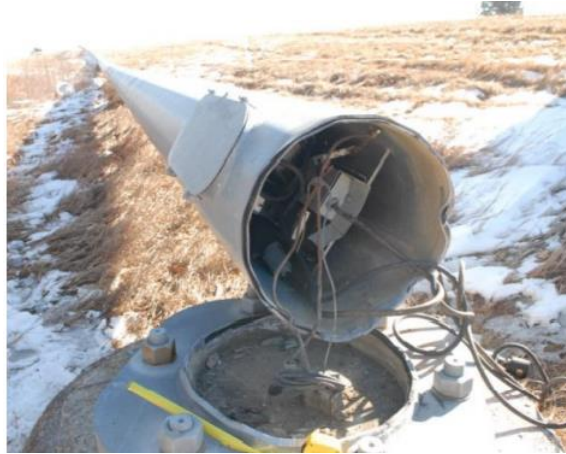
Figure 14. Photo. Failure of high mast lighting tower due to fatigue loading ( Sim et al., 2020 ).
