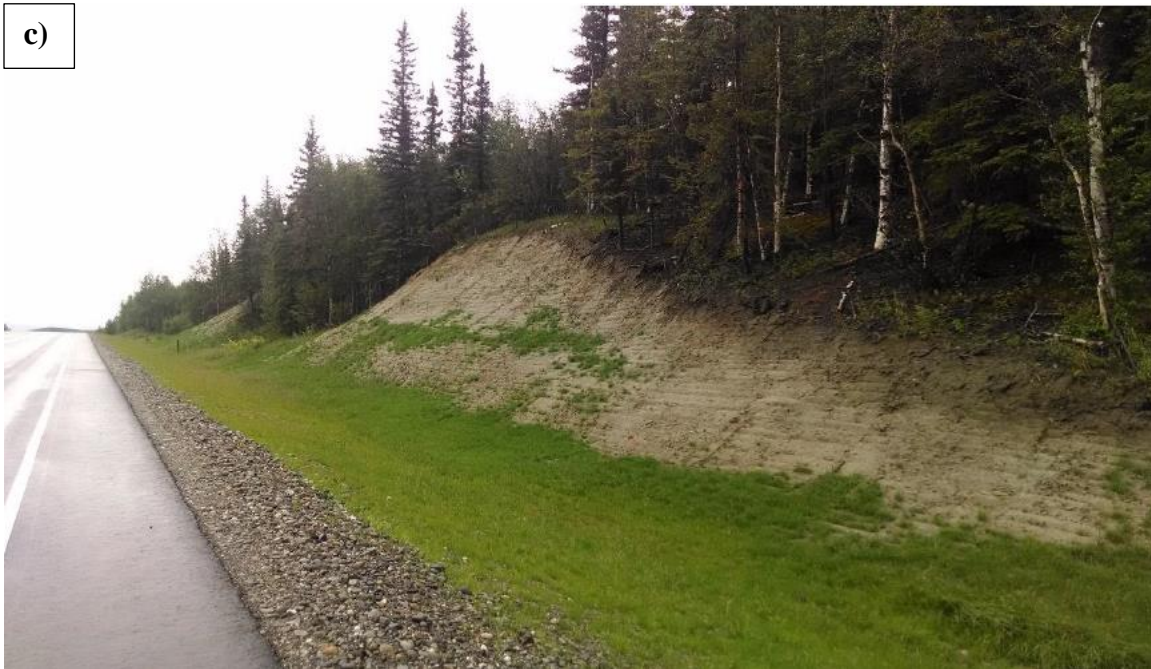
Figure 22. Photo. Class C soil-slope, this geotechnical asset is a stable cut slope showing no signs of unstable performance. Depending on the judgment of the rater, this slope might be excluded from the inventory unless some degree of instability manifests ( Beckstrand et al., 2017c ).
