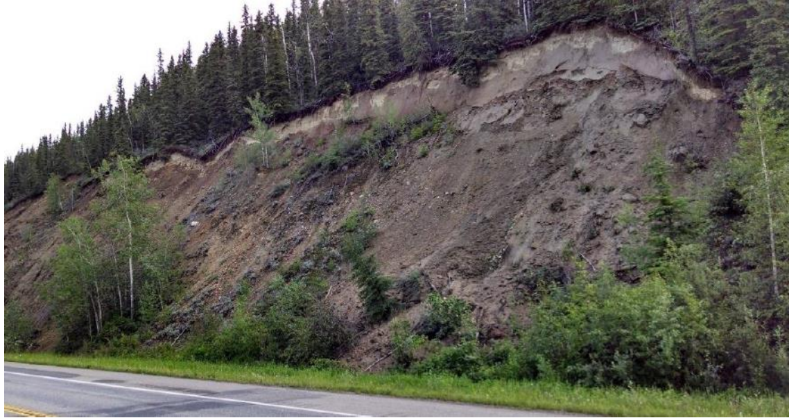
Figure 20. Photo. Class A soil slope, there is an active sloughing of saturated soil and vegetation. This unstable soil slope, due to its height and proximity to the roadway, warrants a detailed examination ( Beckstrand et al., 2017c ).
