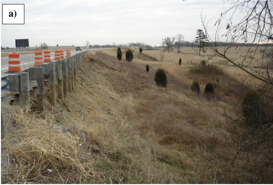
Figure 23. Photo. Example of a Class A embankment-slope: Active sloughing of non-saturated soil and vegetation. This unstable downslope due to its height and proximity to the roadways warrants a detailed examination. Most likely, the head scarp of the translational slide can be seen in the roadway as significant horizontal and vertical deformation. (ODOT, 2013).
