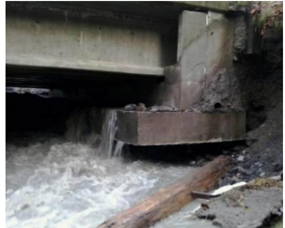
d) Critical condition
