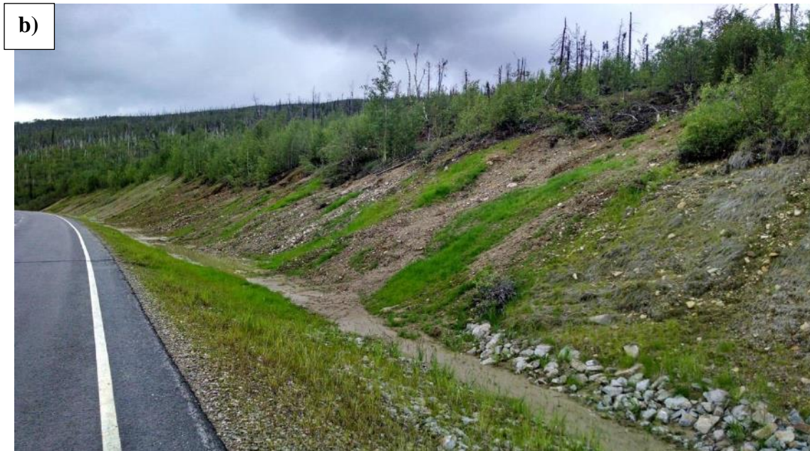
Figure 21. Photo. Class B soil-slope, this cut slope does not represent a safety risk, but the adjacent ditch is filled with debris, and it might require immediate minor intervention from the Operation & Maintenance Office. Roadside ditches should always be clean and obstruction-free to achieve proper drainage conditions. Moreover, a timely report accompanied by a proper condition assessment might prevent a slope from going from a fair condition to a poor one
