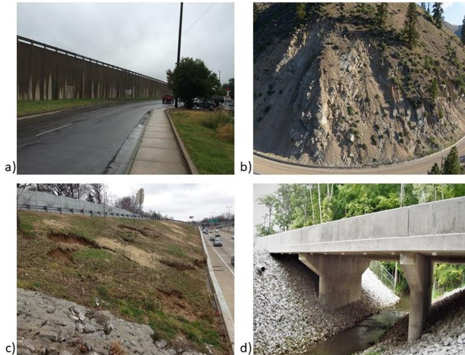
Figure 1. Photo. Examples of different geotechnical assets: a) retaining wall, b) slope system, c) embankment, and d) bridge foundation. Modified from NCHRP (2019).
