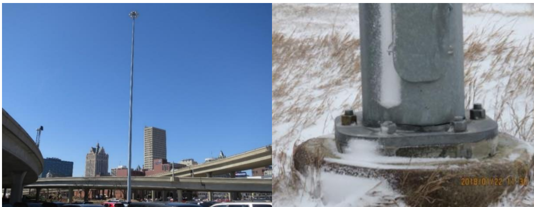
Figure 13. Photo. Examples of high mast lighting tower. ( https://dot.nebraska.gov ).
