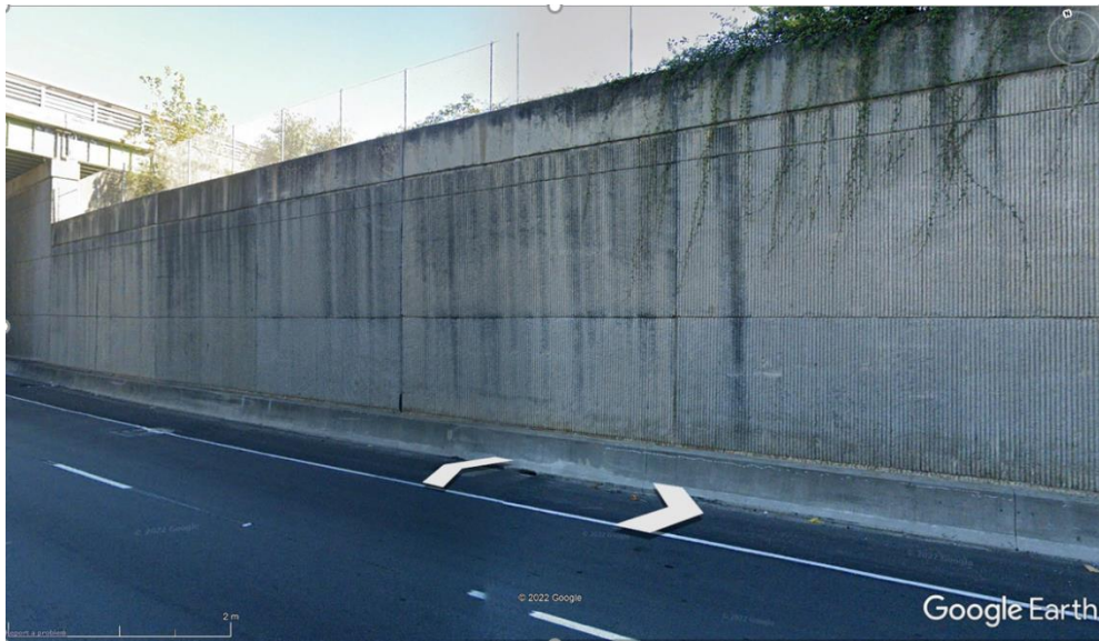
Figure 69. Photo. FN Case, missing retaining wall between RW-02 and RW-03.
