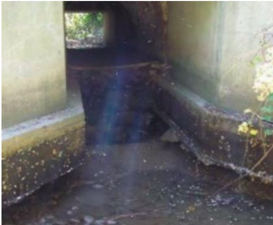
c) Poor condition
