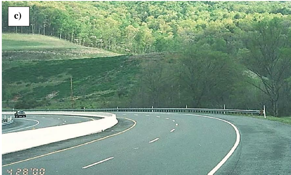
Figure 25. Photo. Example of a Class C embankment-slope: Geotechnical asset with a stable engineered fill showing no signs of unstable performance. Depending on the judgment of the rater, this slope might be excluded from the inventory unless some degree of instability manifests. (No author, retrieved 2022).
