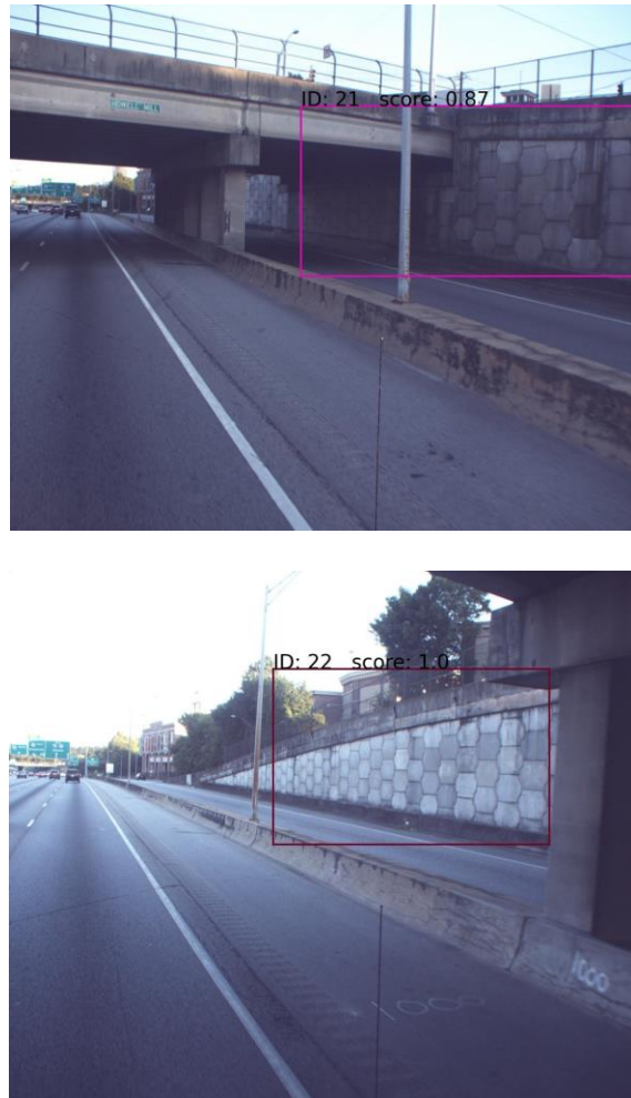
Figure 71. Photo. Examples of double-counted retaining walls due to discontinuity in roadway features (FP case).
