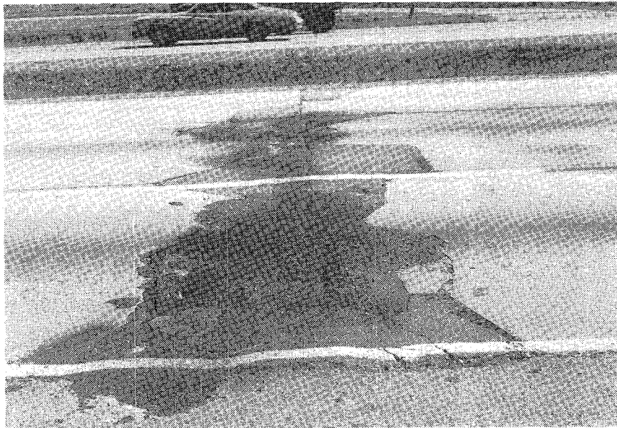
Figure 3.10. Illustration of a joint blowup on a jointed reinforced concrete pavement (JRCP-18, Chicago, Illinois).
