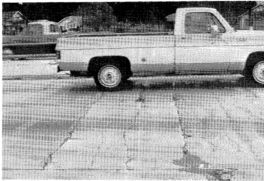
Figure 3.12. Illustration of severe transverse cracking on a continuously reinforced concrete pavement (CRCP-6, Houston, Texas).
