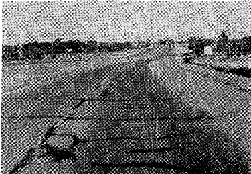
Figure 3.20 Illustration of transverse and longitudinal cracking of flexible pavement (FLEX-4, Minnesota).
