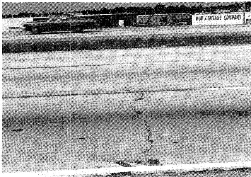
Figure 3.6. Illustration of transverse cracking rated as "major". (JRCP-18-IL).
