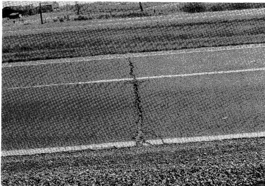
Figure 3.25 Illustration of a severely spalled transverse reflection crack of a composite pavement (COMP-3, Toronto).
