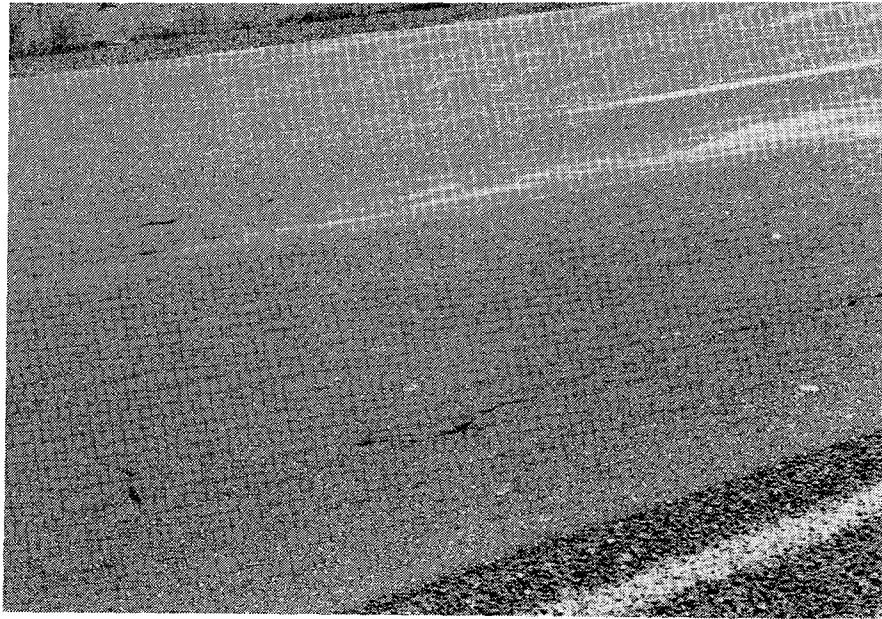
Figure 3.16. Illustration of alligator (fatigue) cracking distress in wheelpaths of flexible pavements (FLEX-17, Arizona).
