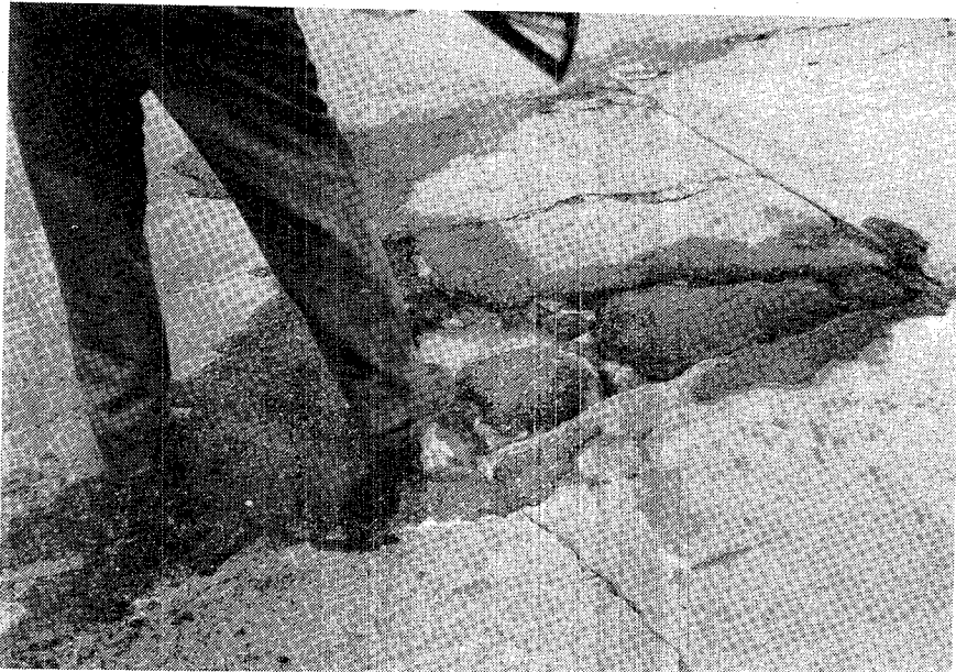
Figure 3.15. Illustration of a localized failure on a continuously reinforced concrete pavement (CRCP-6, Houston, Texas).
