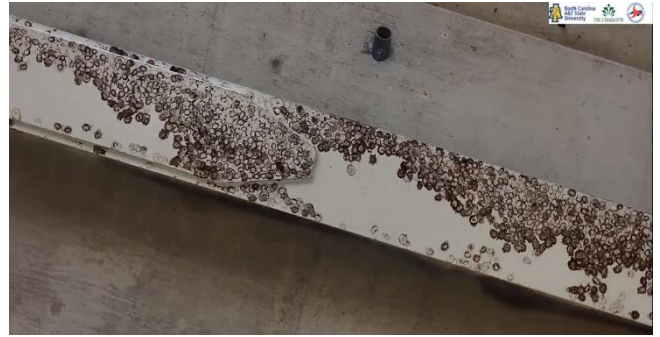
Figure 7.11: Staining on underside of girders.
