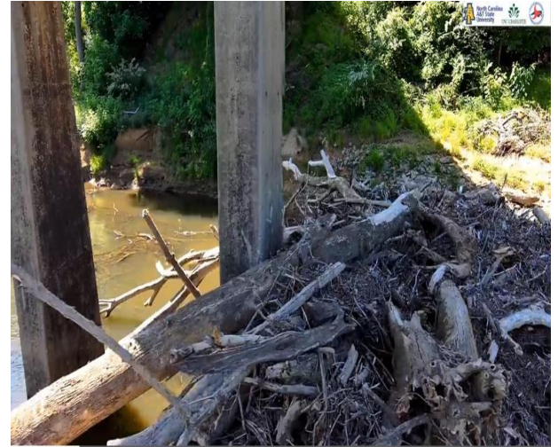
Figure 7.3: Debris pile from high flow event piled against column. Using imaging analysis technology, the volume of the pile could likely be calculated to assist in debris removal activities
