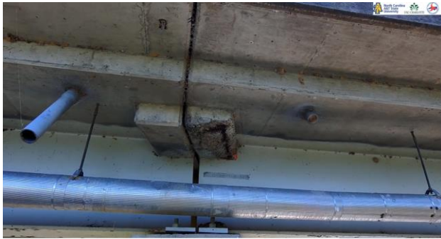
Figure 7.10: Spall with exposed, corroded rebar in concrete diaphragm overhang. Condition of drainage pipes and utility conduit can also be observed.
