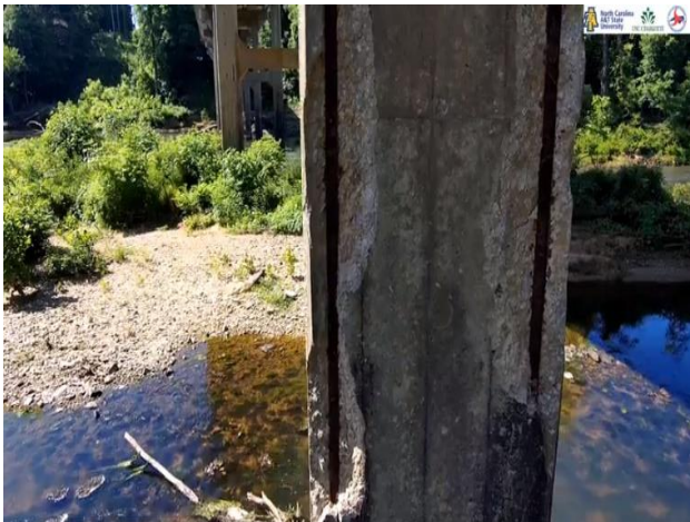
Figure 7.4 Spalls on column, corroded longitudinal steel. At closer magnifications of the image, the deformations on reinforcing bars are visible, as well as cracks alongside the spalled areas. Note the condition of the channel bottom is also evident.
