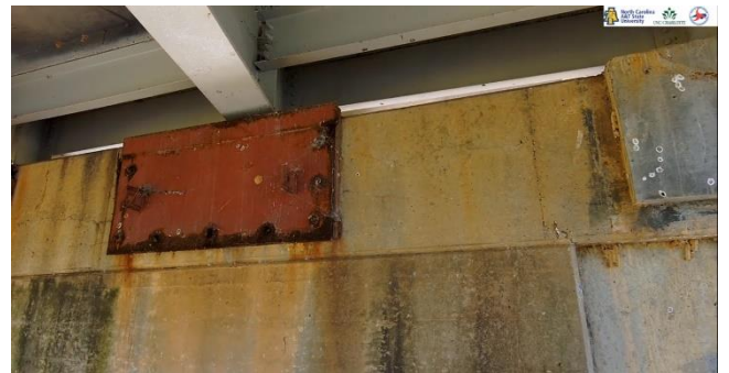
Figure 7.9: Steel plates bolted onto pier cap, with corrosion evident. Condition of girder, diaphragms and connections can also be observed.
