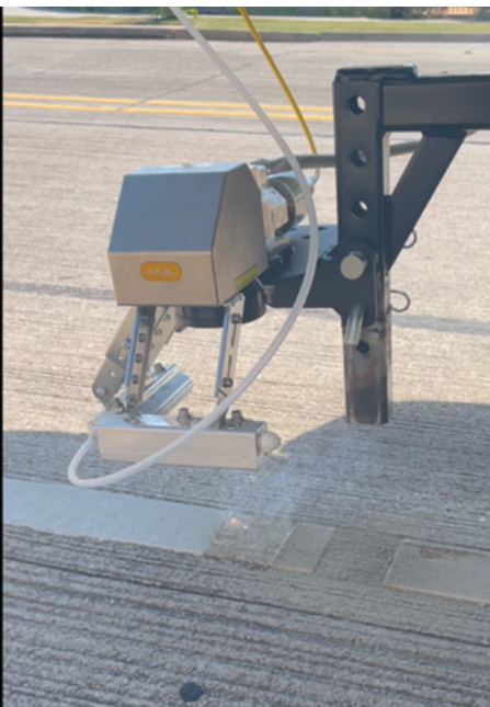
Figure 1. Laser system in operation: white thermo stripe removal from a concrete surface.
