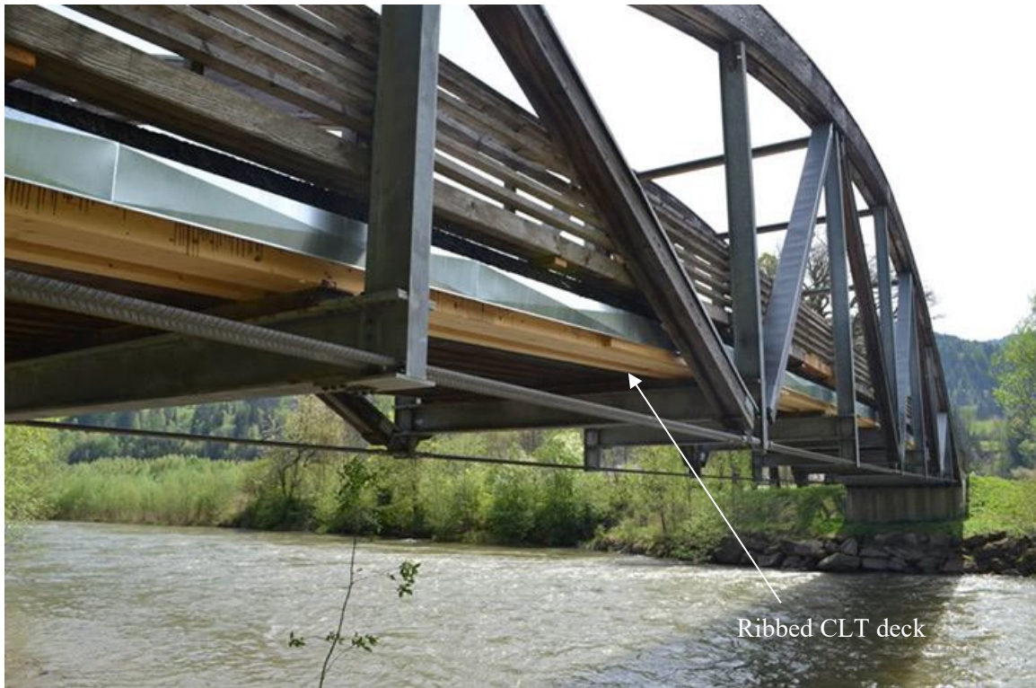
Figure 2.4 Arch bridge with CLT deck over River Mur, Austria (Behrens and Benner 2015)
