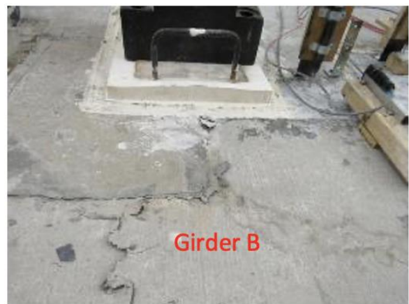
f. LMC Continuous Joint after Testing
