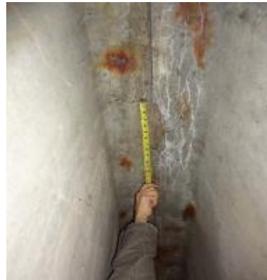
b. Spalling and Corrosion from Underside of a Girder
