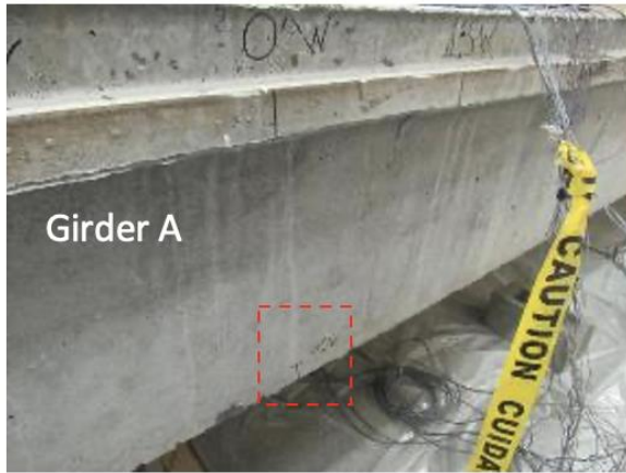
a. First Crack During Loading to 60 kips on West Girder
