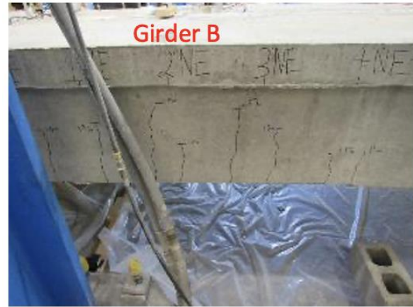
b. East Side of Girder B Damage at 1.5-in. Deflection
