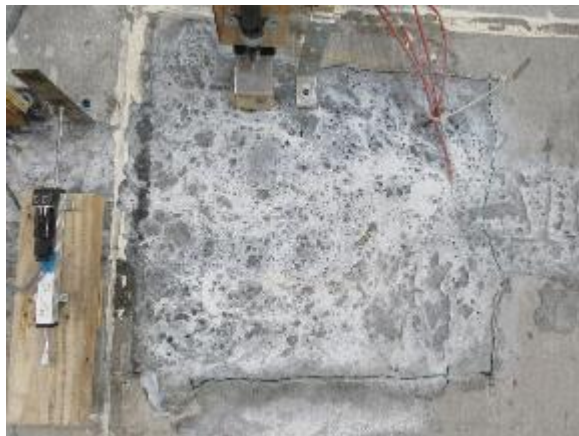
e. UHPC Pocket Joint after Testing
