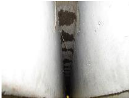
a. Leak in LMC before Testing
