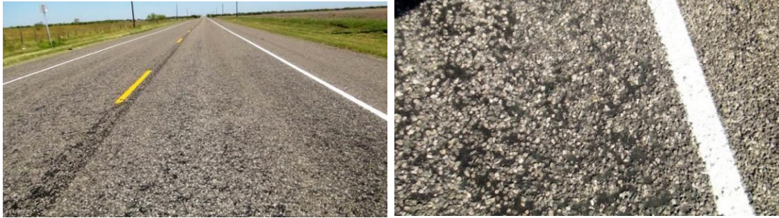
Figure 11. Example of Inadequate Performance on 16-CRP-2 after the First Winter.
