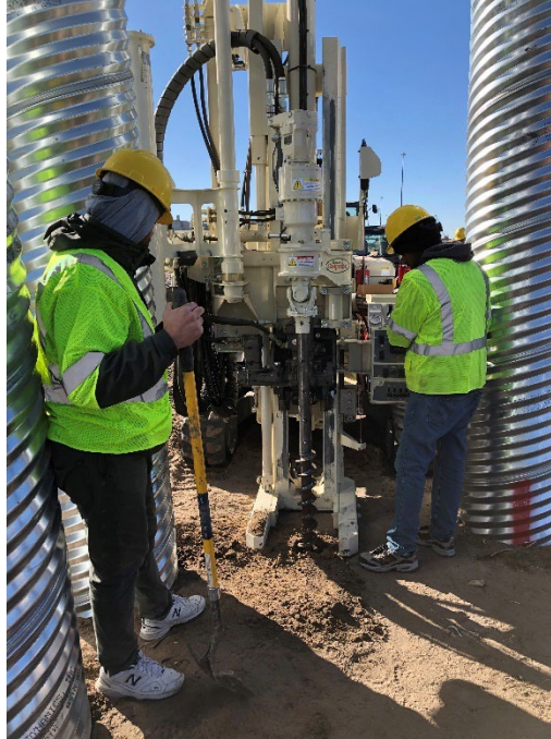
Figure 3.19: Creating Bore Holes in the Foundation Soil using a Drilling Rig Machine
