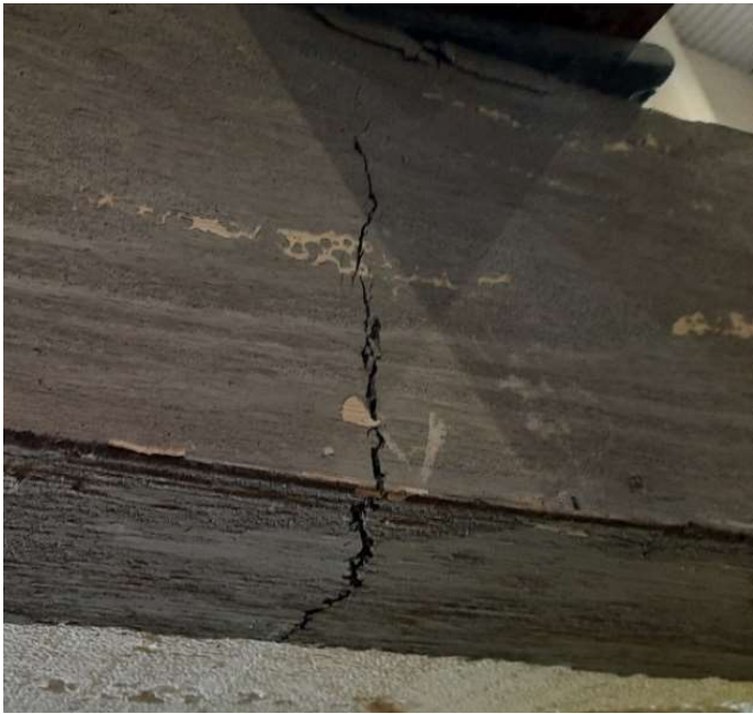
Figure 5.5: Flexure failure mode of the UHPC ribbed slab in positive moment
