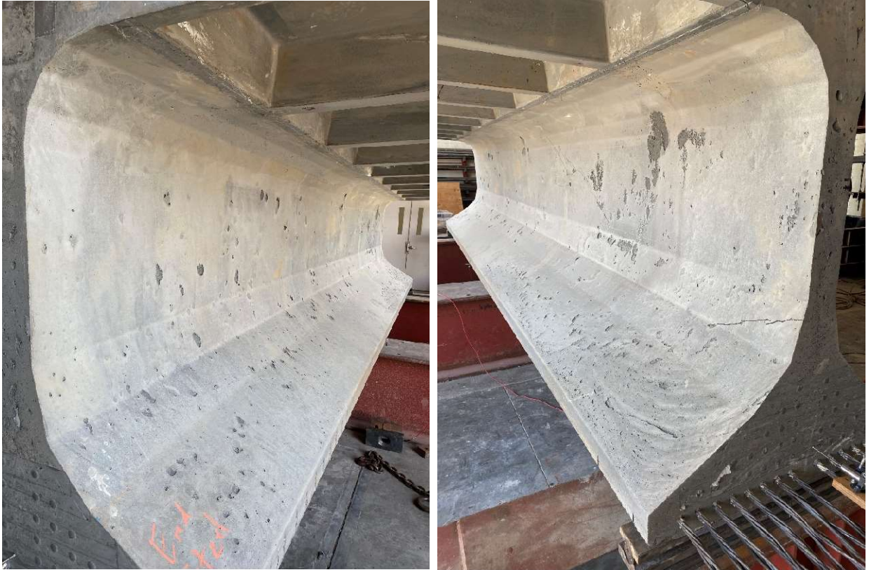
Figure 5.25: End zone cracking at both girder ends
