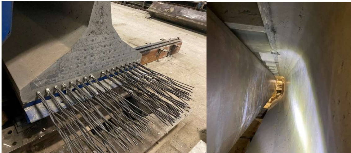
Figure 4.8: Specimen after stripping and prestress release showing girder end (left) and web (right)
