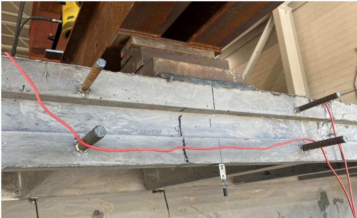
Figure 5.29: Cracking of unreinforced edge rib at early loading
