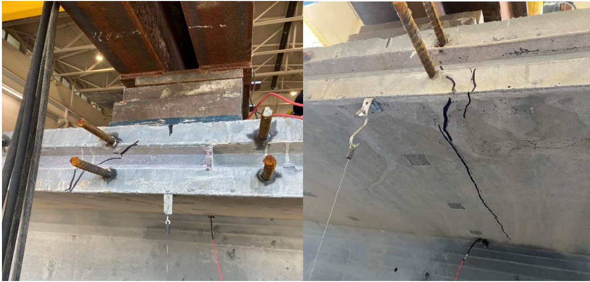
Figure 5.34: Transverse flexure cracks at the side and bottom of the solid slab
