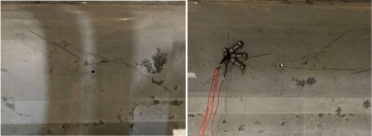
Figure 5.24: Diagonal tension cracks at both girder sides
