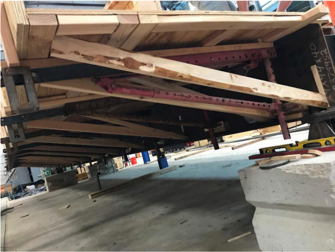
Figure 4.5: Bracing of formwork for the cantilevers. Additional bracing shims were added to help reduce construction deflections.
