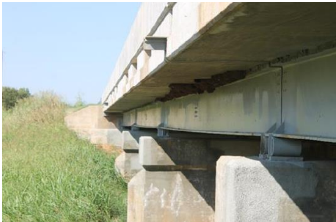
Figure 3.1. SH 14 Over Eagle Chief Creek, Bridge "A", Woods Co., Oklahoma. View lkg South
