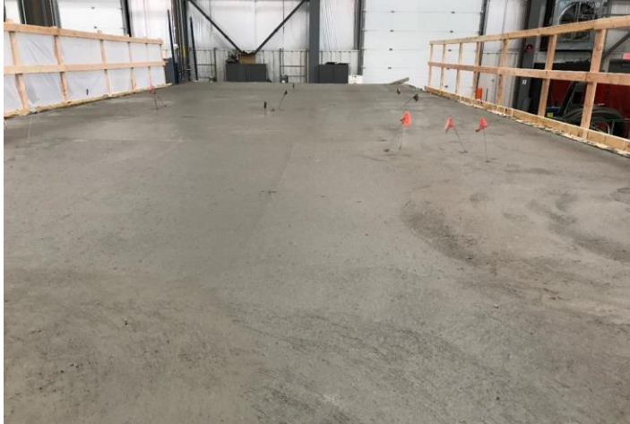
Figure 4.13: Bridge deck after casting and finishing concrete. A broom finish was applied.
