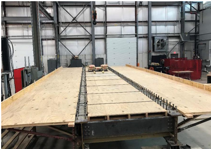
Figure 4.3: Formwork being prepared for casting the bridge deck on the prototype bridge
