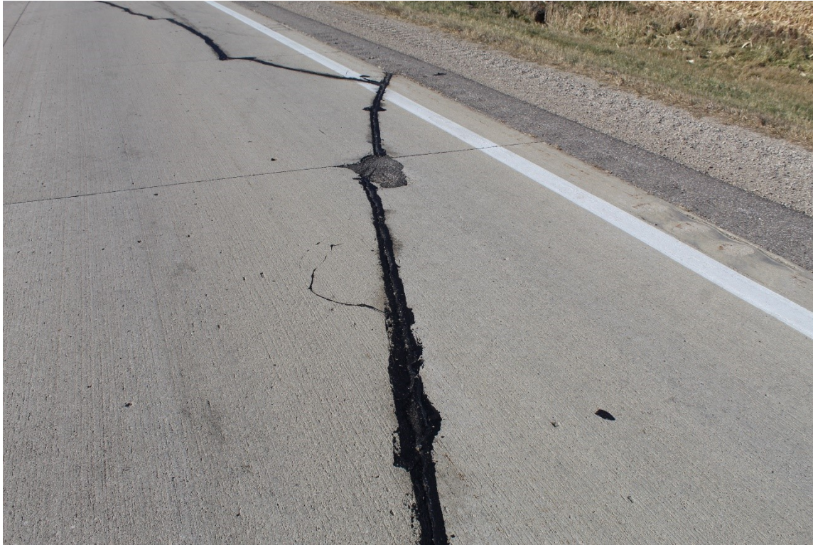
Figure 2.10 Longitudinal crack with spalling at intersection with transverse joint near location of dowel bars
