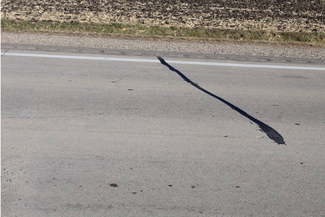
Figure 2.11 Transverse crack on CSAH 46
