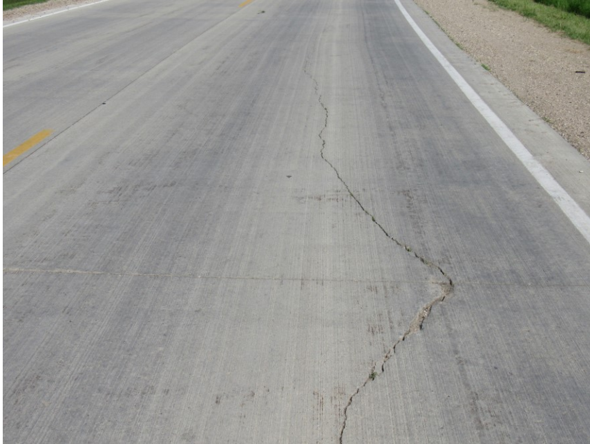
Figure 2.33 Longitudinal cracking on a COA overlay on a different section of CSAH 46 in Freeborn County, MN
