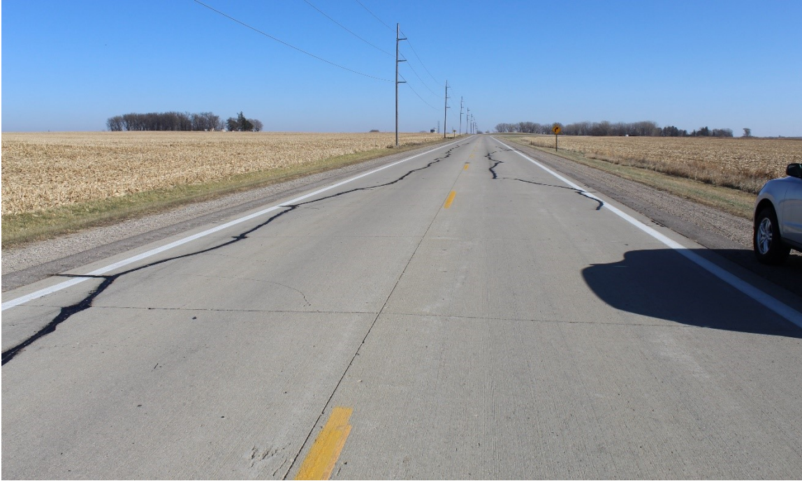
Figure 2.8 CSAH 46 typical project conditions showing longitudinal cracking
