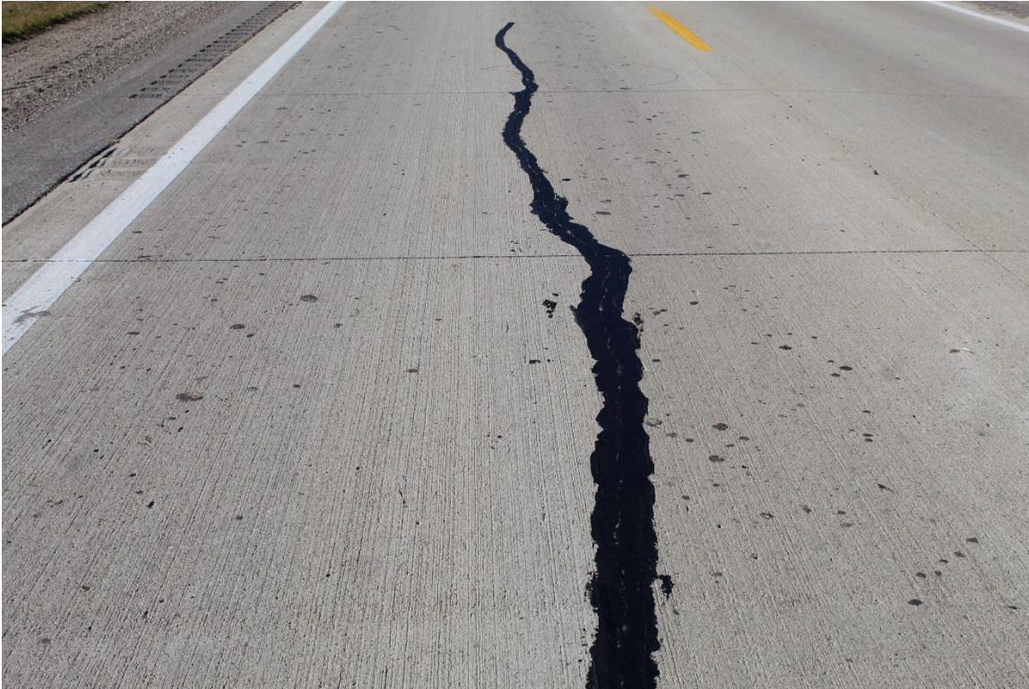
Figure 2.9 Close-up view of longitudinal crack filled with sealant
