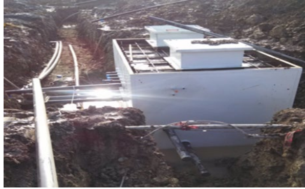
Figure 7. Horizontal Geothermal Trenches and Well Field Control Vault
