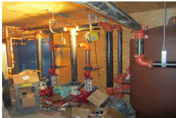
Figure 6. Heat Exchange Control Facility
