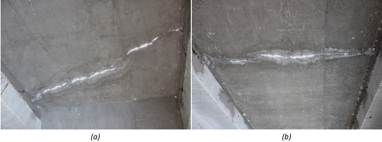
Figure 5.5 Full-depth cracks in steel-reinforced bridge deck (27W36)
