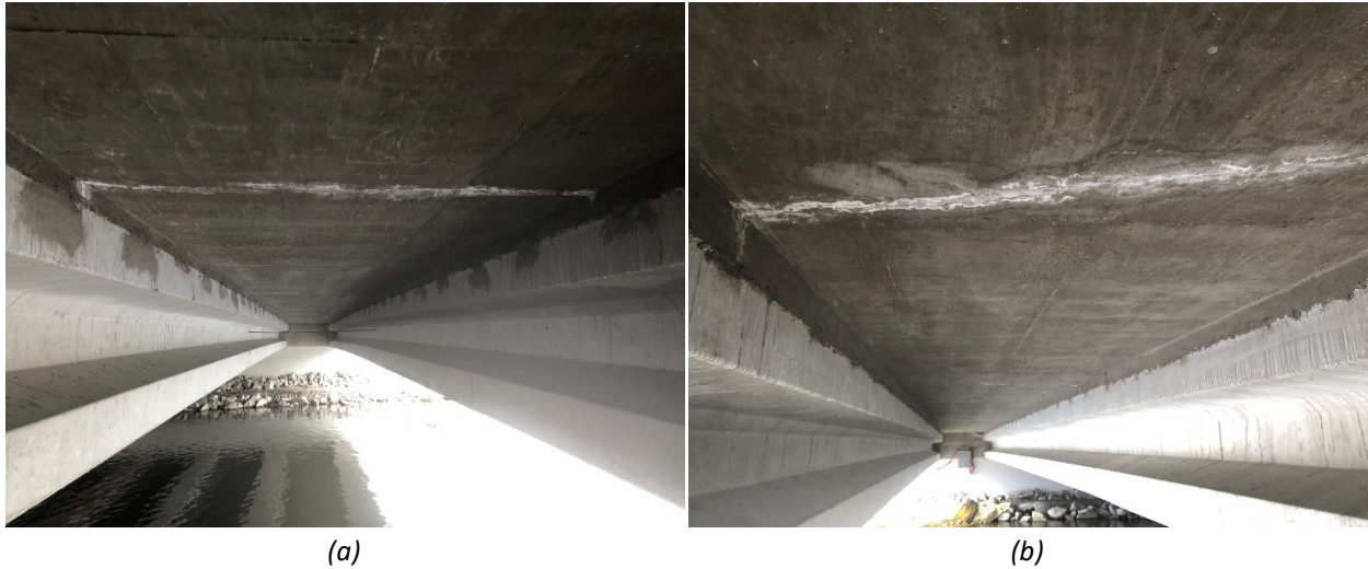
Figure 5.2 Full-depth cracks in the bridge decks: (a) steel-reinforced bridge deck (27W36) and (b) GFRP-reinforced bridge deck (27W37)
