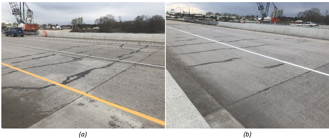
Figure 5.1 Top surface cracks in the bridge decks: (a) steel-reinforced bridge deck (27W36) and (b) GFRP-reinforced bridge deck (27W37)
