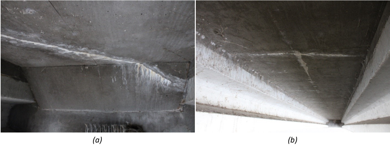
Figure 5.4 Full-depth cracks in GFRP-reinforced bridge deck (27W37)
