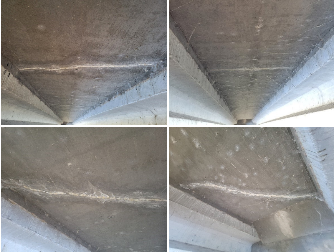
Figure 5.7 Cracks on the bottom surface of GFRP-reinforced bridge deck (27W37)
