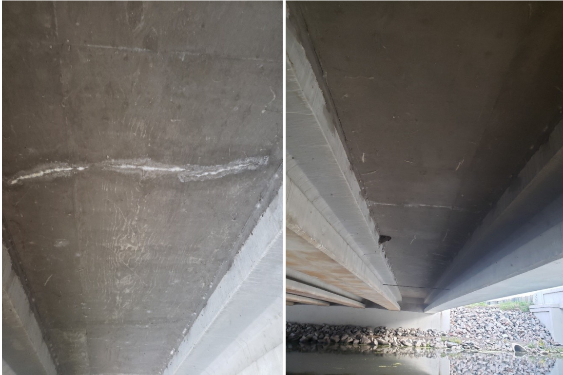
Figure 5.6 Cracks on the bottom surface of steel-reinforced bridge deck (27W36)
