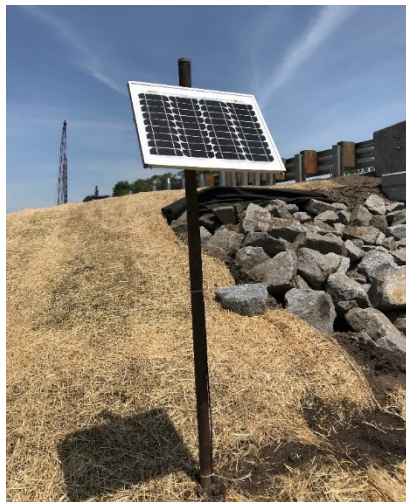
Figure 3.6. Solar panel installed at the bridge site
