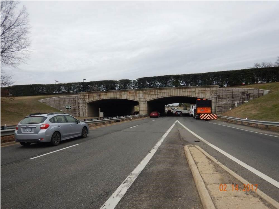
Figure 7. Stone Masonry Veneer on a Concrete Rigid Frame Bridge in an Urban Setting, 1945 (Arlington County Structure No. 5020)
