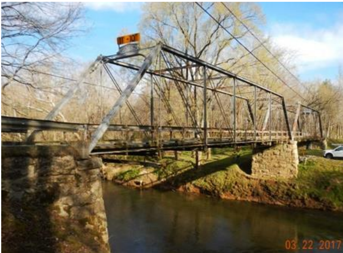
Figure 1. Stone Masonry Piers and Abutments Supporting an 1884 Truss Bridge (Brunswick County Structure No. 6104)
