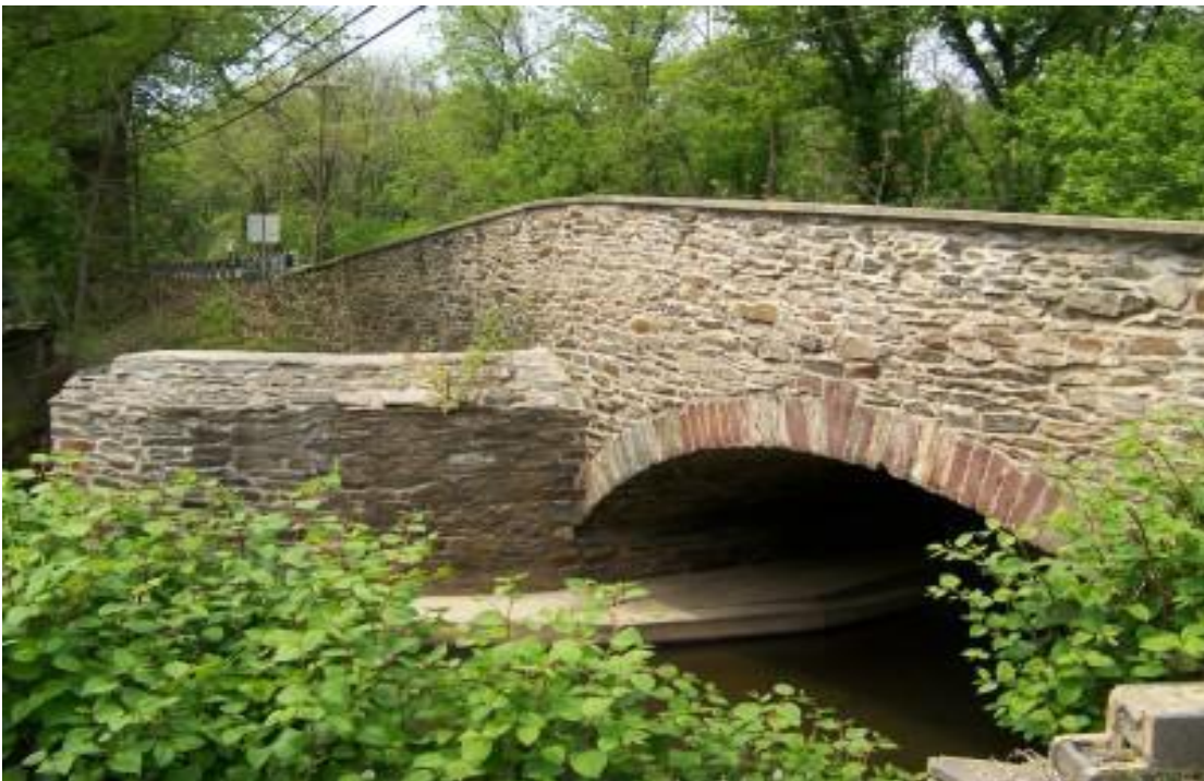
Figure 5. Stone Masonry Arch, Built as a Turnpike Bridge in the First Quarter of the 19 th Century (Loudoun County Structure No. 1025). A contrasting color of stone was used in the voussoirs for decorative effect. Note the relatively flat arch that is seen in many stone masonry bridges of this era.
