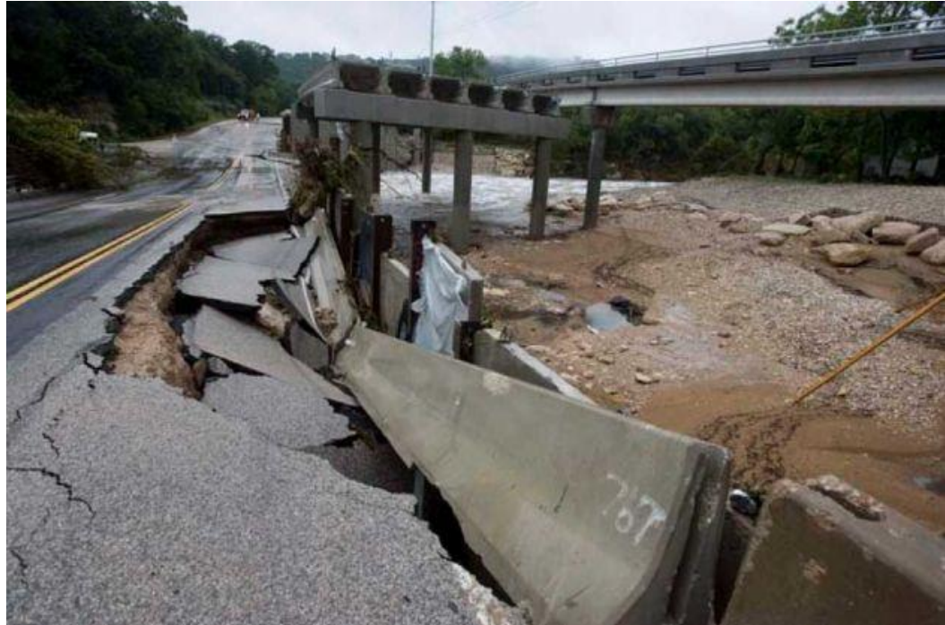
Figure D-14 Damage to RM 2222 at the Bull Creek Crossing Due to Overnight Flooding September 7-8, 2010 (Tropical Storm Hermine)
