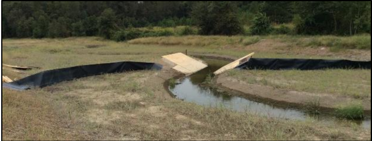
Figure 8. Image of the trapezoidal wooden section and the floodplain curtain at CLMD during construction
