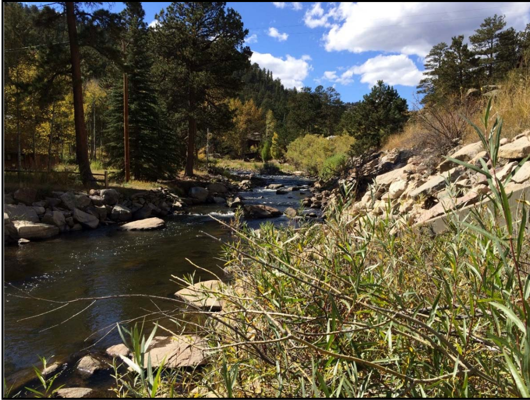
Figure 7: Armored Embankment along the Big Thompson River at the Culvert Outlet. Photograph provided courtesy of FHWA.
