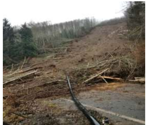
Figure 2. A 2021 slide near Clallam Bay covered 325 feet of the highway. Source: WSDOT.
