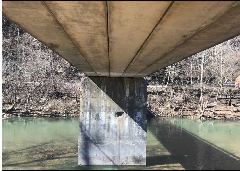
Figure 2. Prestressed concrete box beam bridge with expansion joints suitable for bat use (Photo by Copperhead Consulting).
