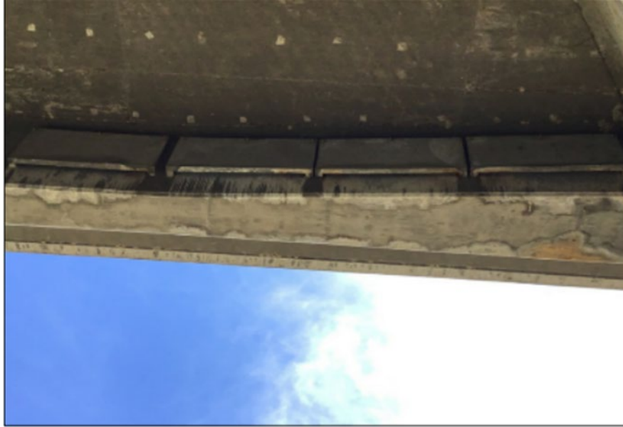
Figure 9. Concrete Oregon wedge style bat habitat with urine staining from Yuma myotis and Mexican free-tailed bats. (Photo used with permission from H.T. Harvey & Associates and HDR 2021)
