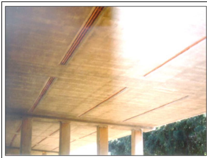
Figure 7. Photo of recessed cast-in-place roost boxes from Caltrans Bat Mitigation: A Guide to Developing Feasible and Effective Solutions. (Photo used with permission from H.T. Harvey & Associates and HDR 2021)
