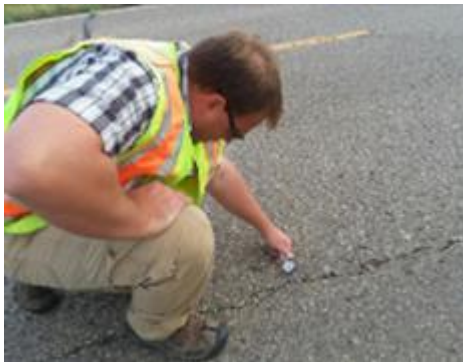
Figure 7: CRACK MEASUREMENTS WITH CALIPER
