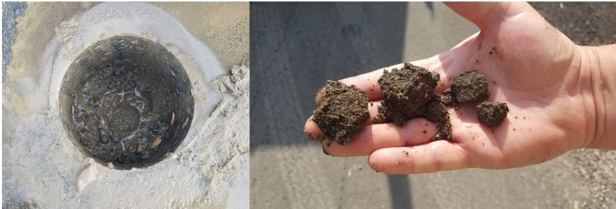
Figure 3-4 Core Hole and Material Obtained from BASE ONE® Section (Hubbard CSAH 46) at C-4.
