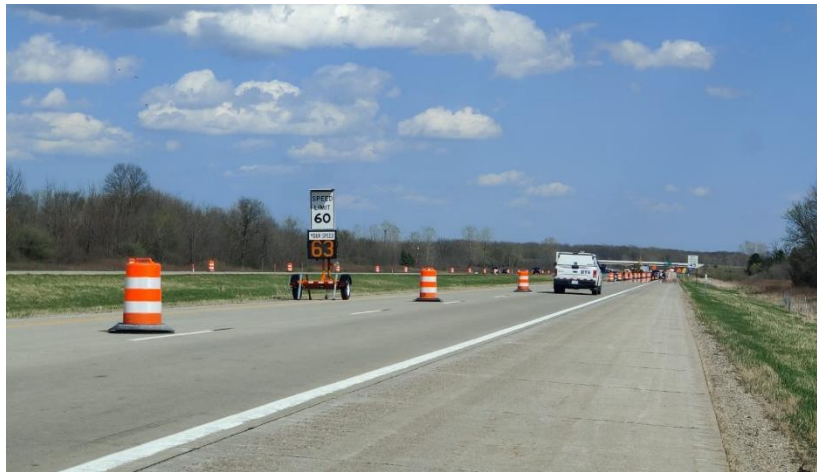
Figure 10. Speed feedback trailer positioned at the end of taper at WB I-69 work zone
