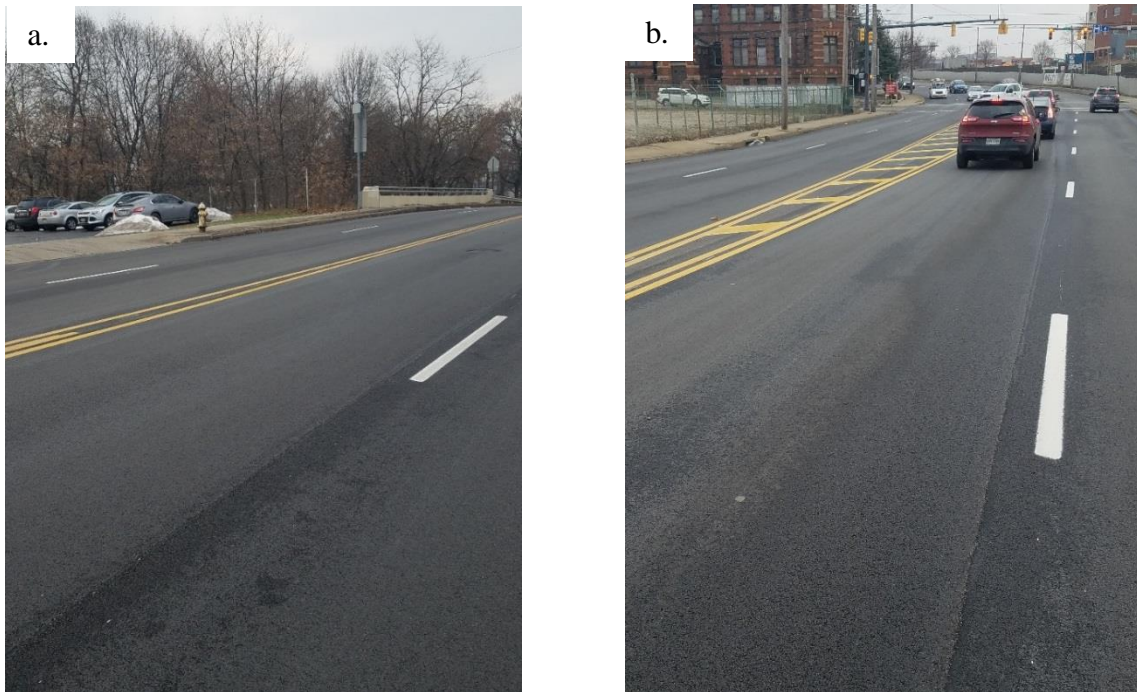
Figure B.22 Pictures of Akron Test Sections after Two Months of Construction: a) Control polymer Section, b) Lehigh Rheopave GTR Section
