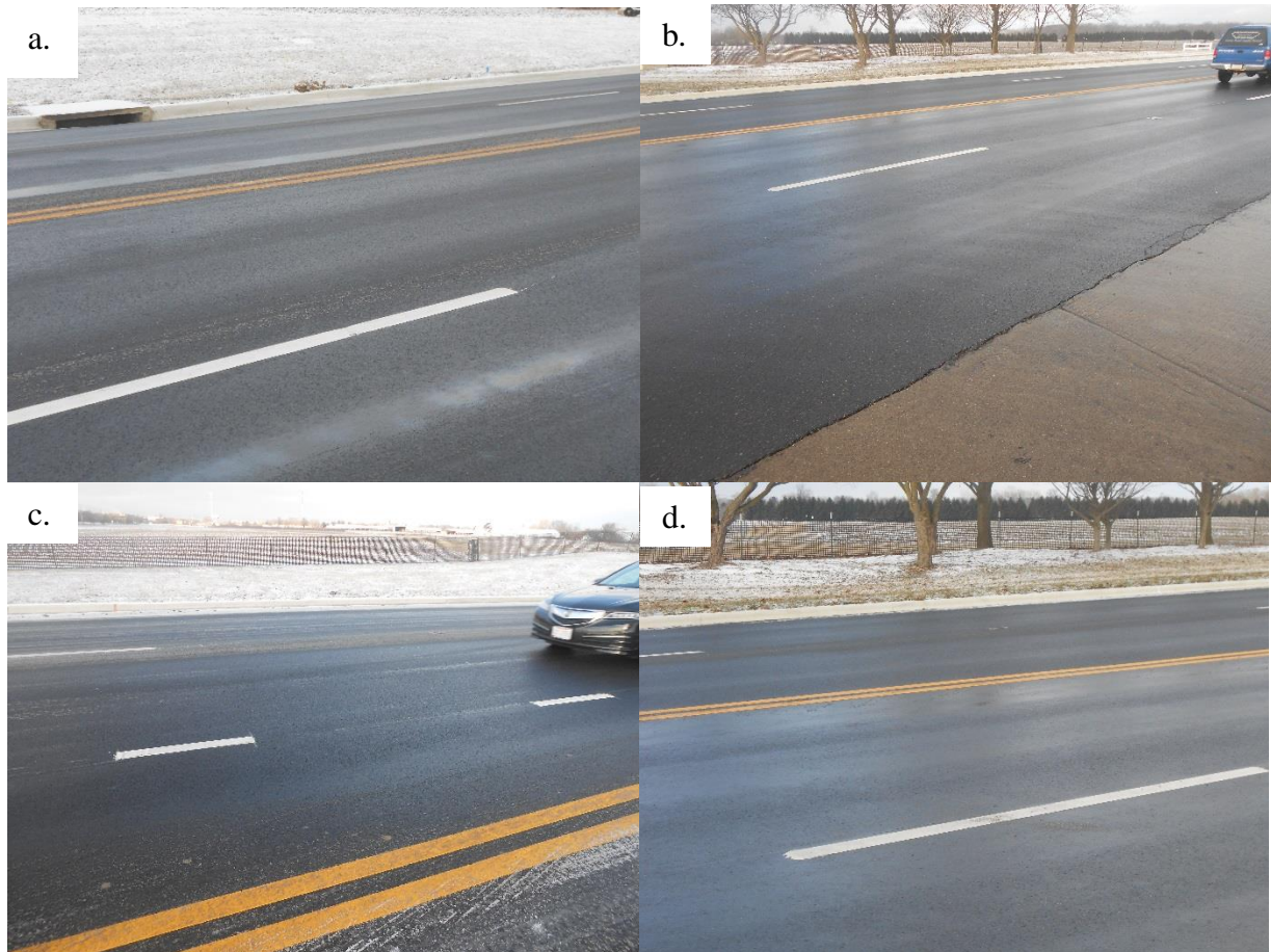
Figure B.20 Pictures of Columbus Test Sections after Five Months of Construction: a) Control polymer Test Section, b) Lehigh GTR Section, c) Lehigh Rheopave GTR Section, and d) Liberty GTR Section
