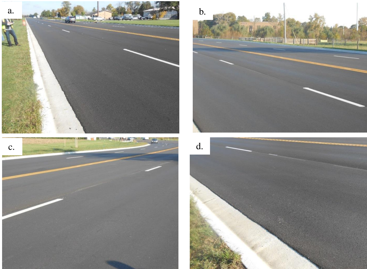
Figure B.19 Pictures of Columbus Test Sections after Two Months of Construction: a) Control polymer Test Section, b) Lehigh GTR Section, c) Lehigh Rheopave GTR Section, and d) Liberty GTR Section
