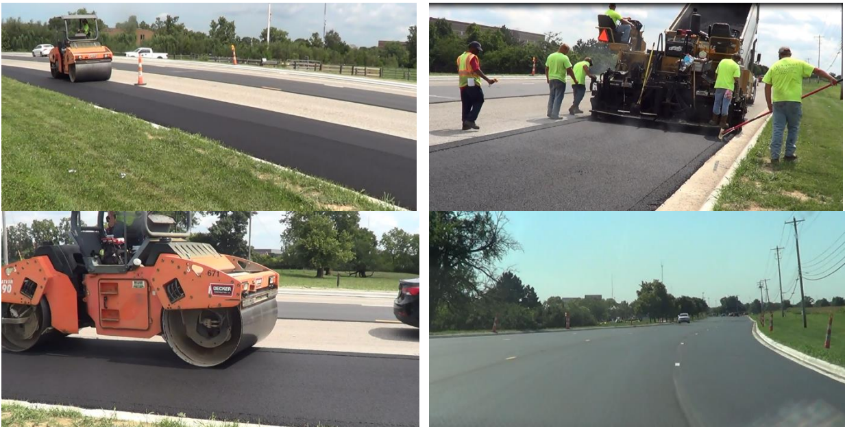
Figure A.2 Pictures Taken during Construction of Test Sections in the City of Columbus.
