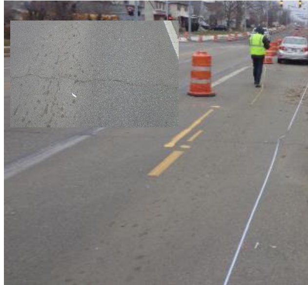
Figure 3.7 Pictures of GTR Modified Pavement Sections on Smithville Road after 2.5 Years of Service
