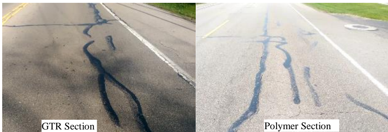
Figure 3.3 Pictures of GTR and Polymer Modified Pavement Sections at King Road After 10 Years Of Service
