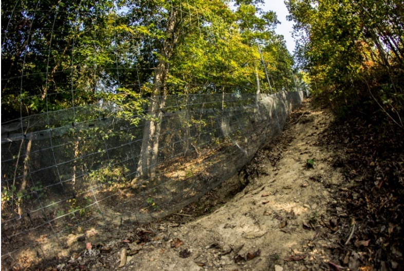
Figure 7-11. Damage to the snake fence. Top: corrosion damage, Middle: tree fall damage, Bottom: erosion damage.
