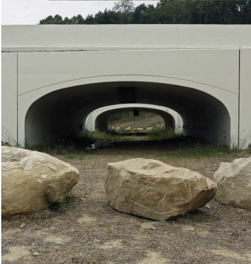
Figure 2-33. Images of Wildlife Underpass 2 (UP2) for large wildlife use, along the U.S. 33 Nelsonville Bypass in Hocking County, Ohio. UP 2 is 125 ft. across with a bottom width of 35 ft. and a maximum height of 9 ft. Aerial photo of UP2 (top) and ground photo (bottom).
