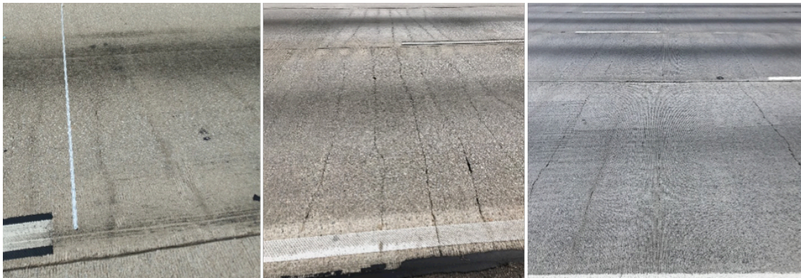
Figure 86 – The Density of Transverse Cracks in Sites 1, 3, and 5
