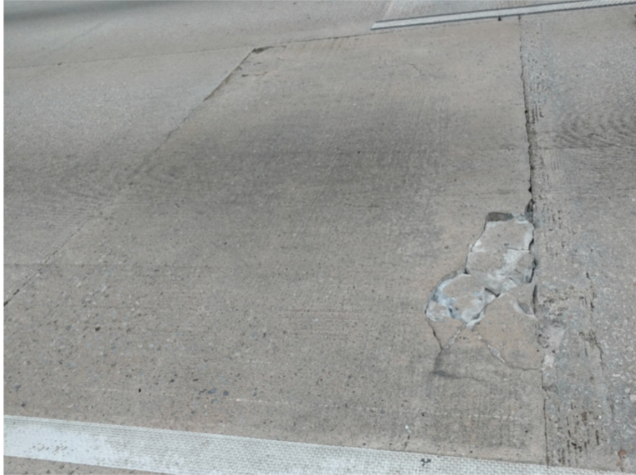
Figure 48 – A Patched Area of the Outside Lane at S3-b
