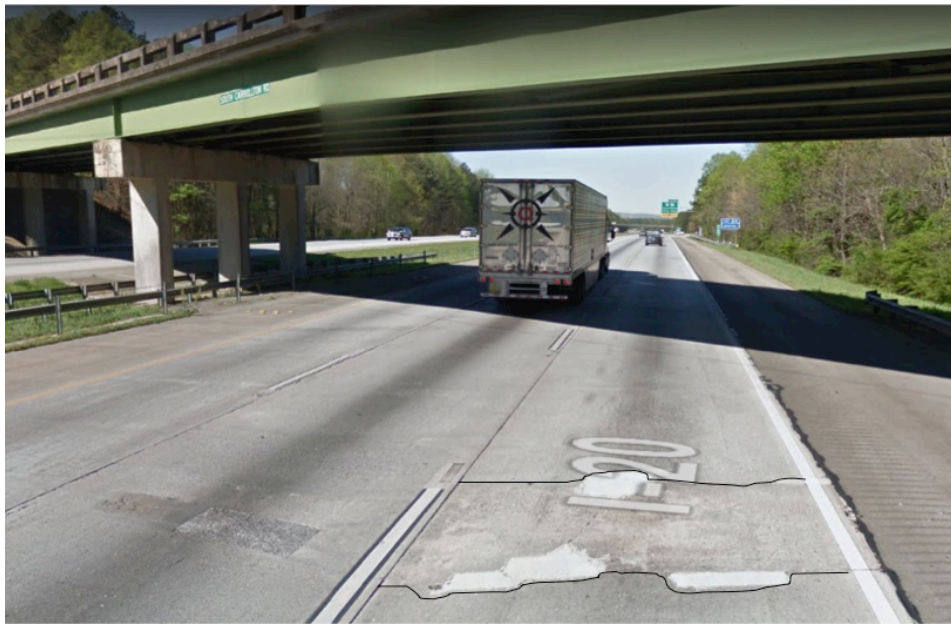
Figure 51 – A Patched Area of the Outside Lane at S3-d (Google Maps, 2017)
