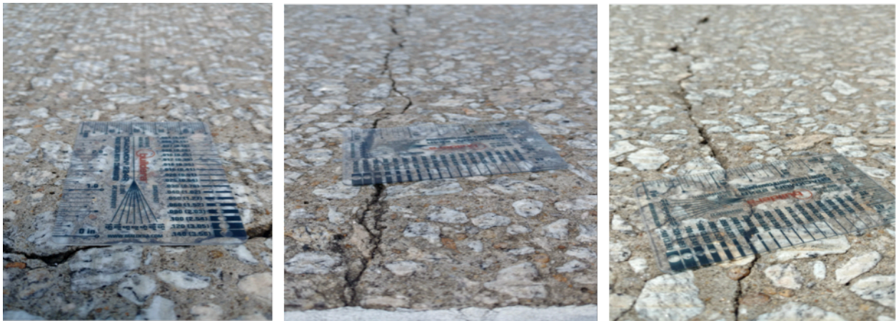
Figure 30 – Crack Width Measuring at S1-b, S1-c, and S1-d
