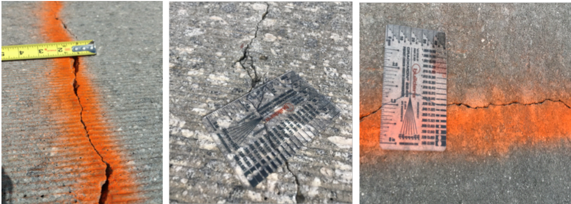
Figure 61 –Sample Crack Widths at S4-a and S4-c
