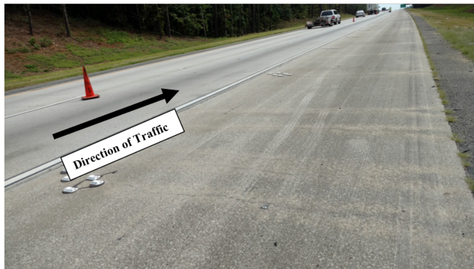
Figure 38 – Typical Cluster Transverse Cracks Pattern at (a) S2-a and (b) S2-c
