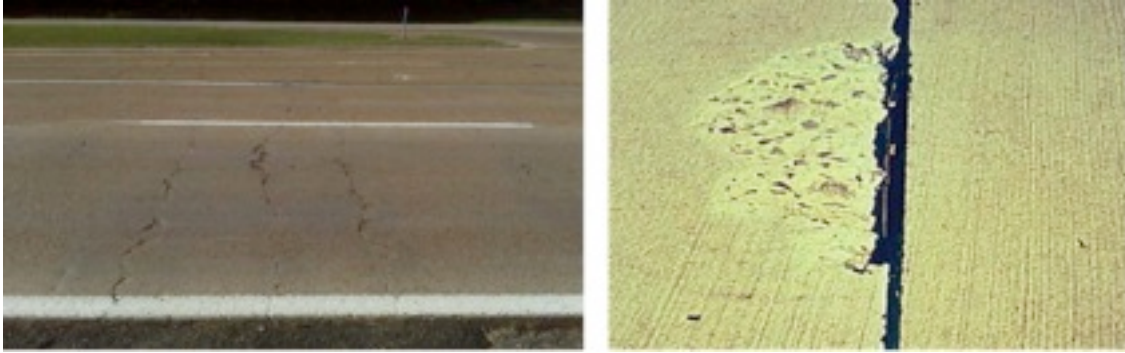
a. Spalling at Transverse Cracks
