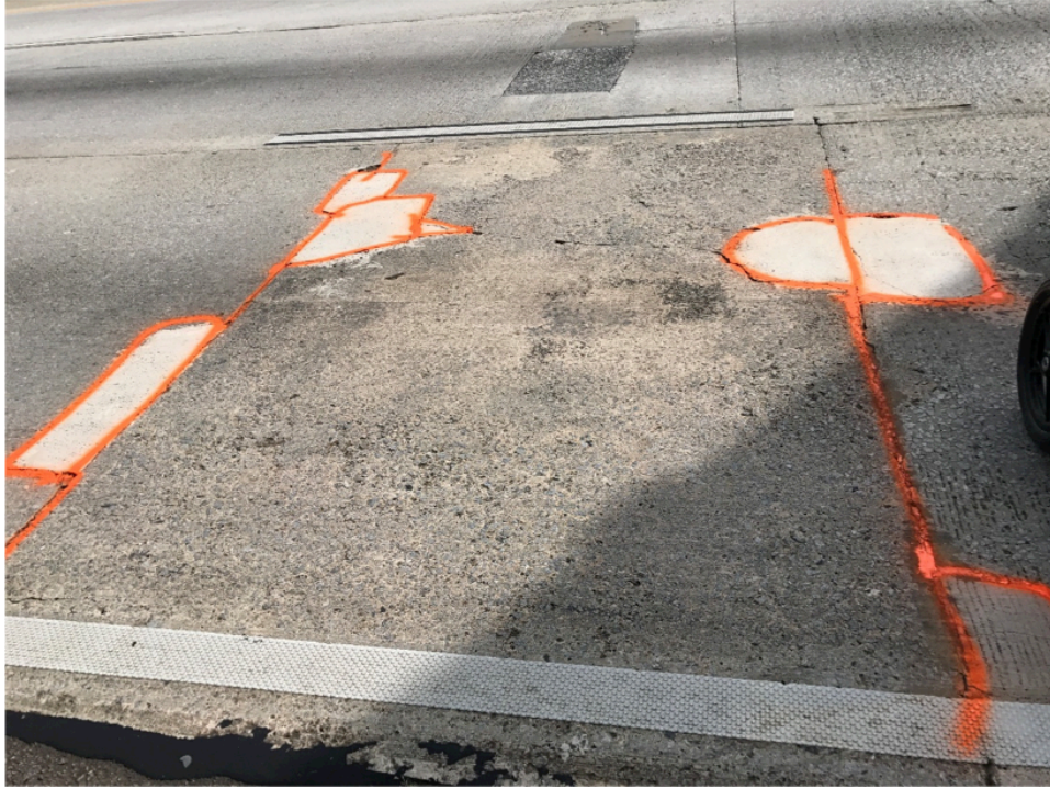
Figure 50 – A Patched Area of the Outside Lane at S3-d
