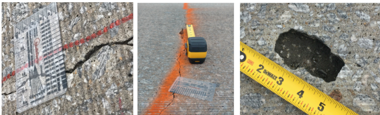
Figure 39 – The Measurement of Crack Widths at S2-a and S2-c
