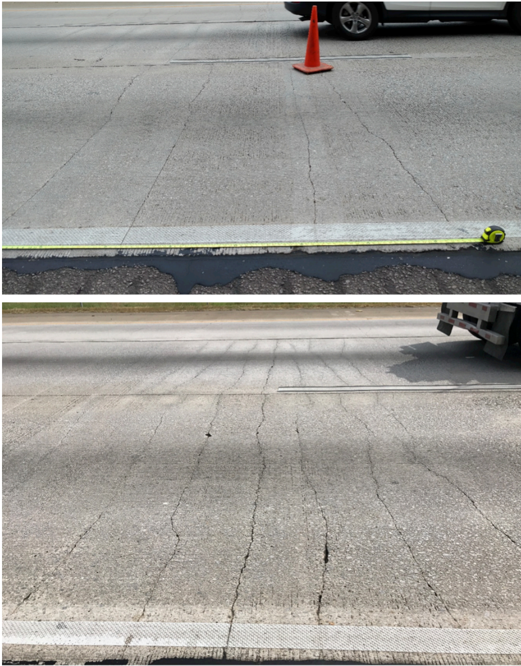
Figure 46 – Typical Cluster Transverse Cracks Pattern at S3-a and S3-c
