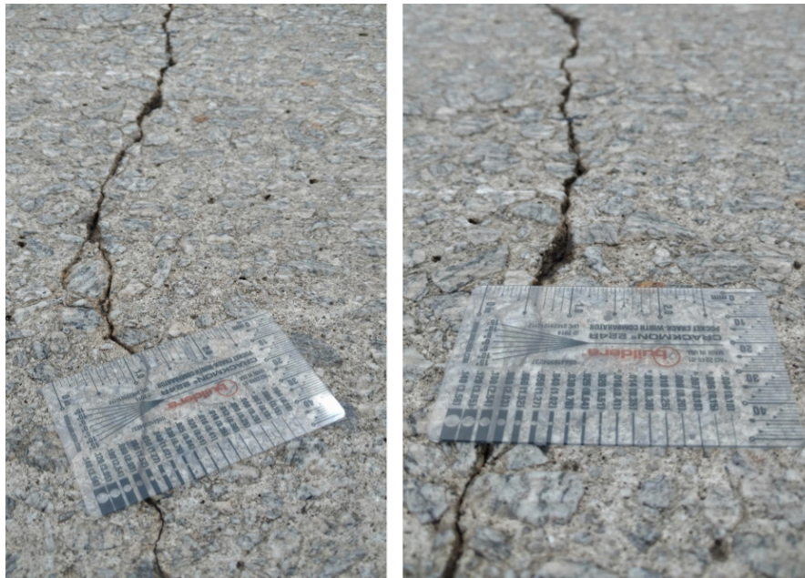
Figure 47 –Crack Width Measuring at S3-a
