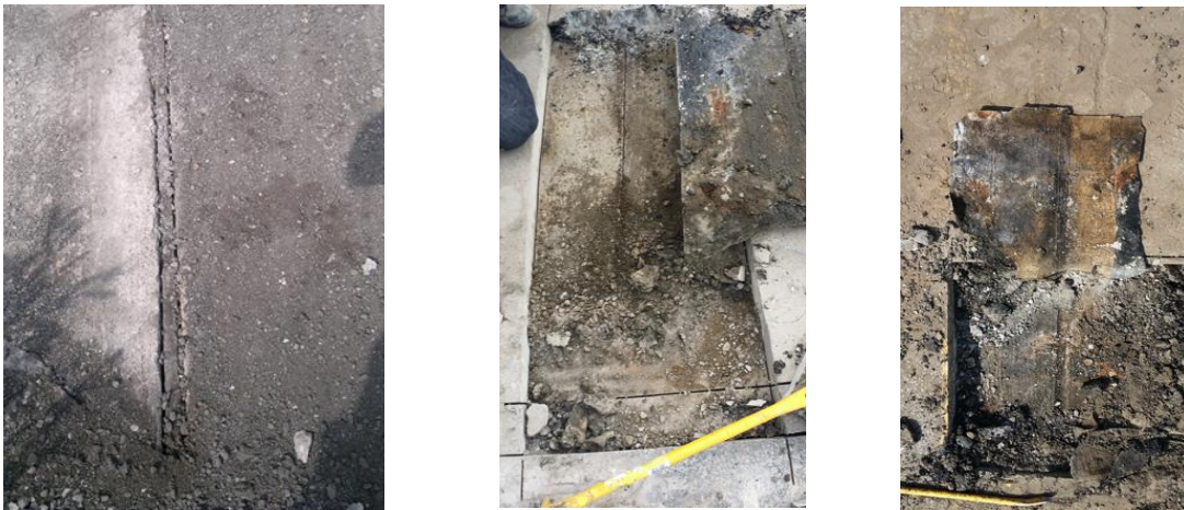
Fig. C.5 Condition of a Typical Joint and Deck Surface
