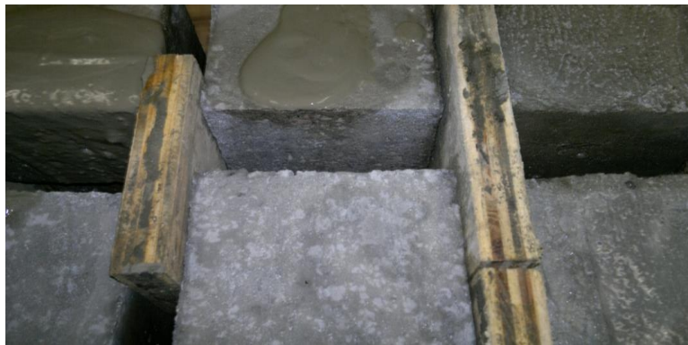
Fig. D.7 Application of Cement Slurry (See on the Left Facing Side)
