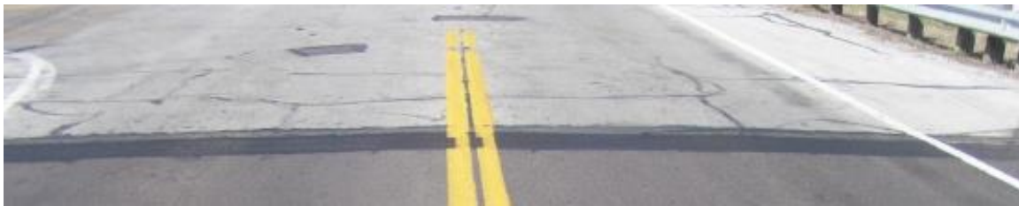
Fig. A.21 One Year after Replacement
