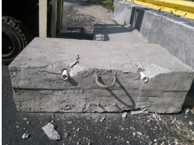
Fig. H.12 Typical Failure in Concrete Units
