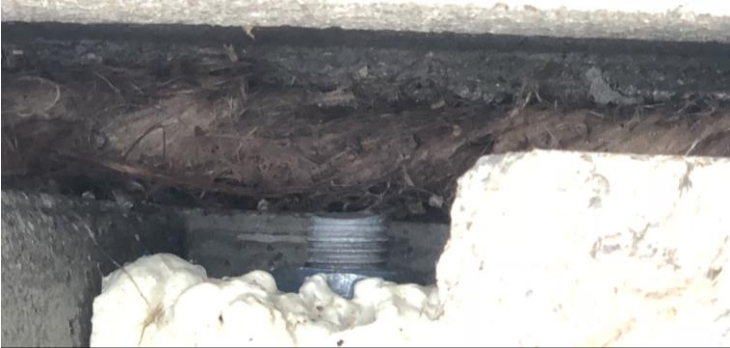
Fig. J.5 Jute Rope Used to Seal the Bottom of the Key Way
