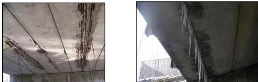
Fig. 2 Severe Deterioration of Underside of ODOT Box-beams at the Longitudinal Joints Due to Corrosion and Spalling (Left) and PennDOT Documentation of Leakage (Right)
