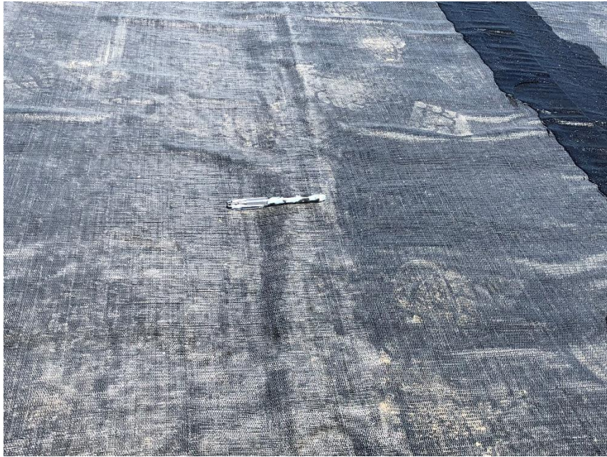
Fig. J.8 Membrane Over Adjacent Beams That were not Level
