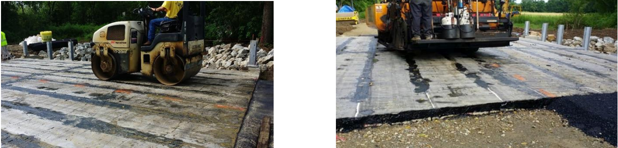
Fig. C.7 Heavy Equipment Being Driven over an Unprotected Membrane
