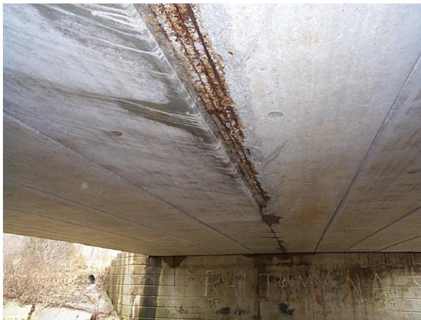
Fig. A.19 Box Beam Deterioration
