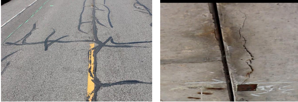
Fig. C.2 Surface Cracks and Path of Truck Wheels ( left ) and Typical Cover Spalling on Bottom Surface ( right )
