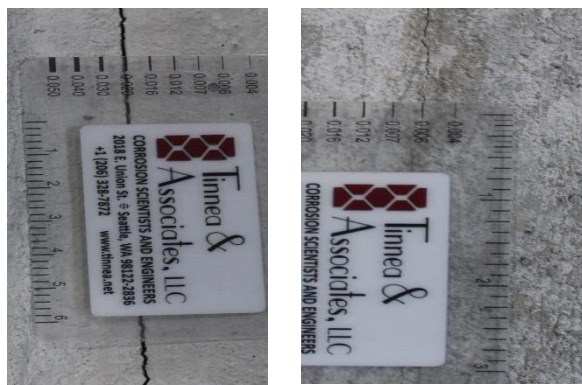
Fig. F.5 Shrinkage Cracks for Set # 1 (Left) – for Set # 2 (Right)
