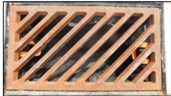
(f) catch basin grate
