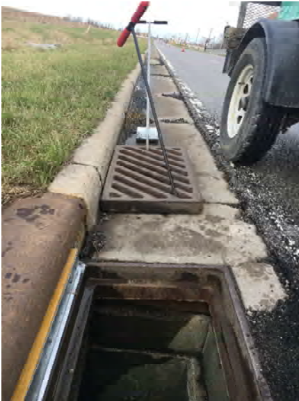
Gutter is in poor condition with patching Downstream Curb
