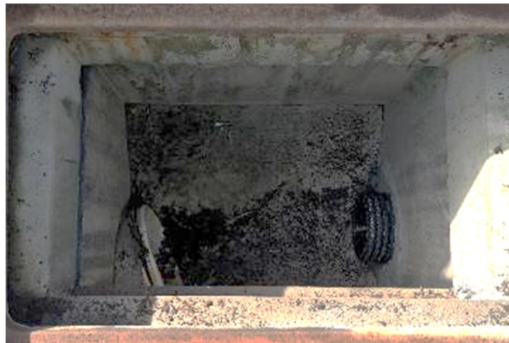
Figure 4-10 Catch Basin Connecting Conduit
