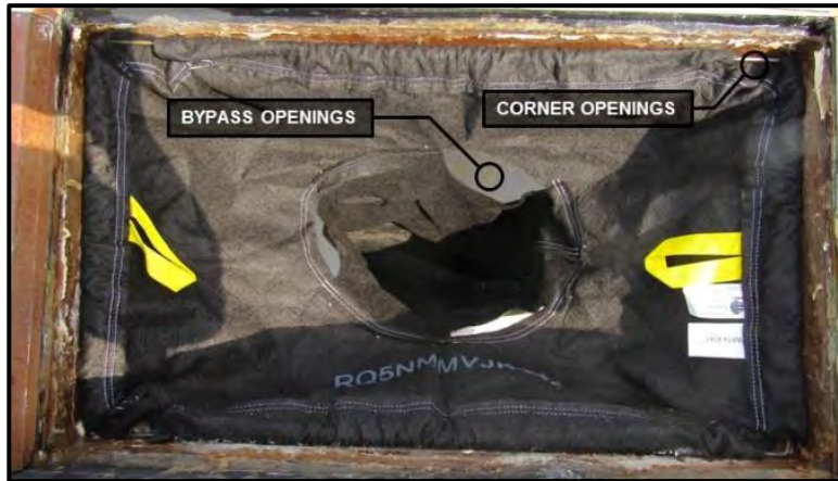
Figure C-15: Openings in Storm Sentinel® allow untreated bypass.
