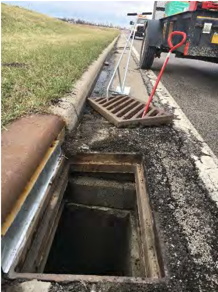
Gutter around CB in poor condition Downstream Curb
