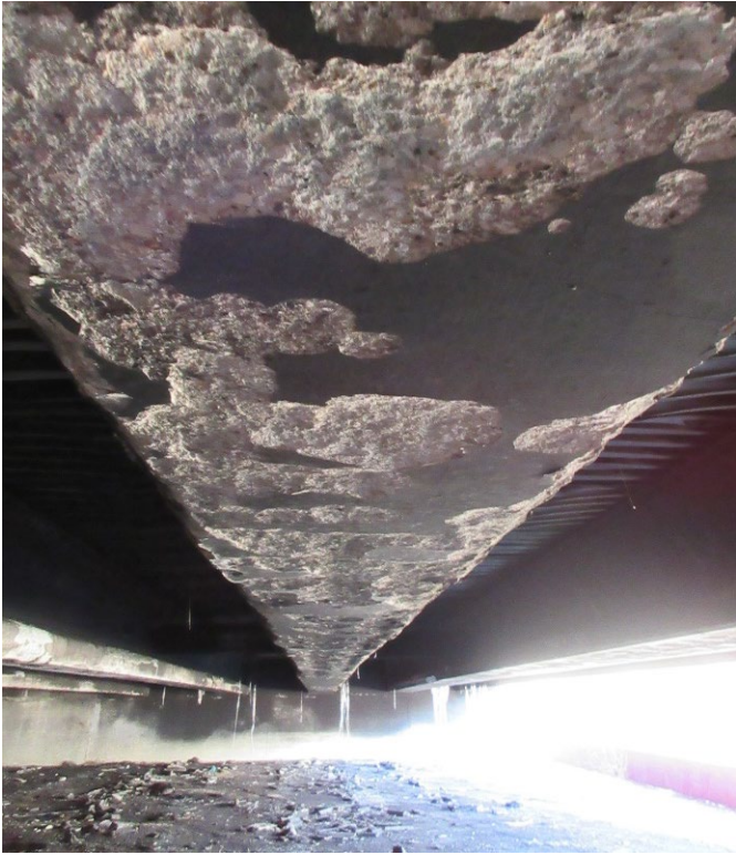
Figure 2. Concrete spalling on concrete girder
