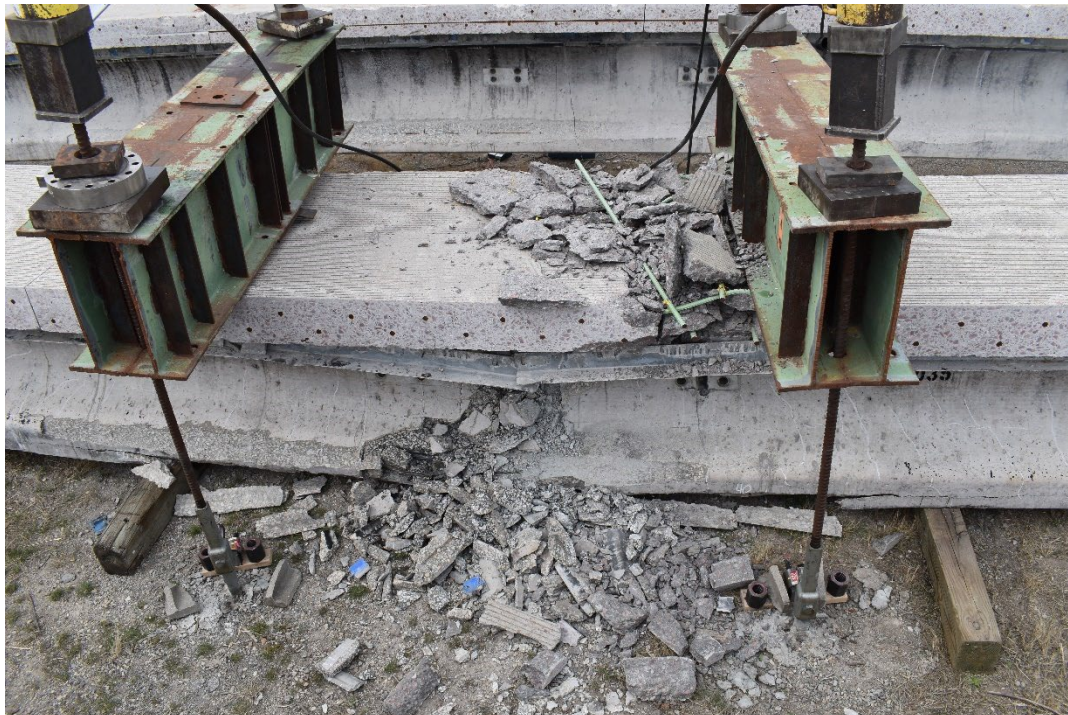
Figure 59. Girder E after failure at midspan
