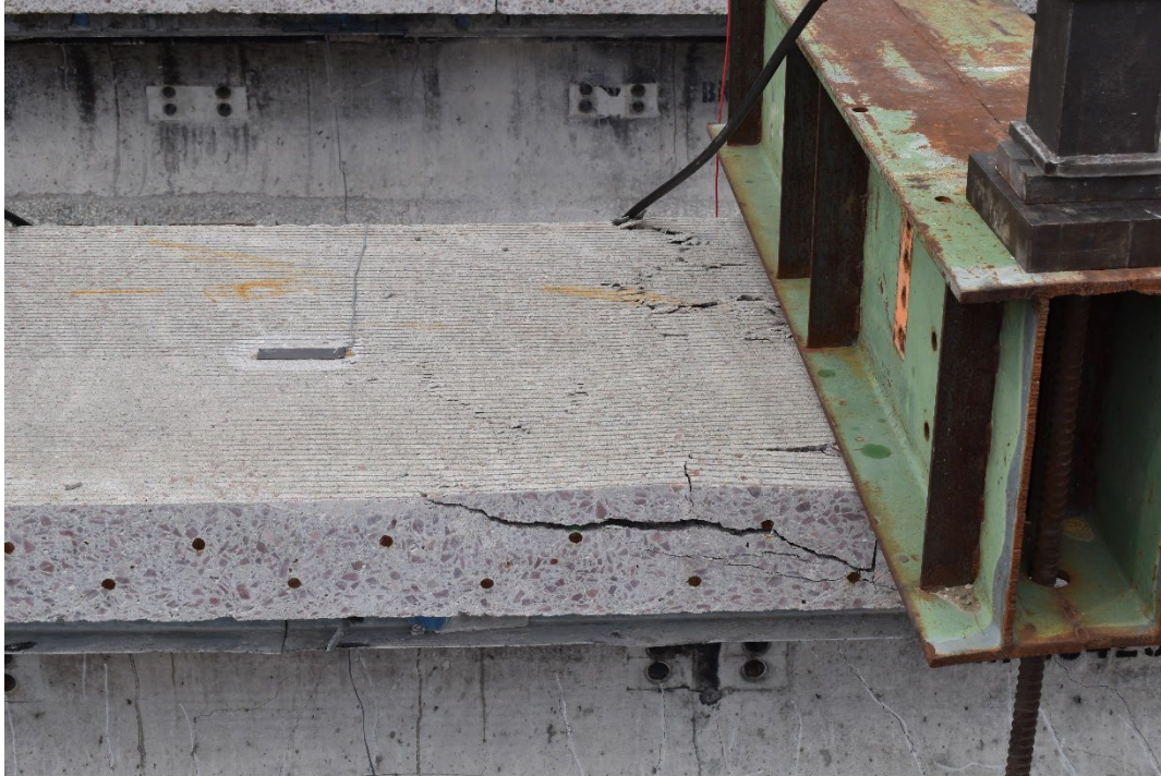
Figure 58. Initiation of deck cracking at Girder E midspan
