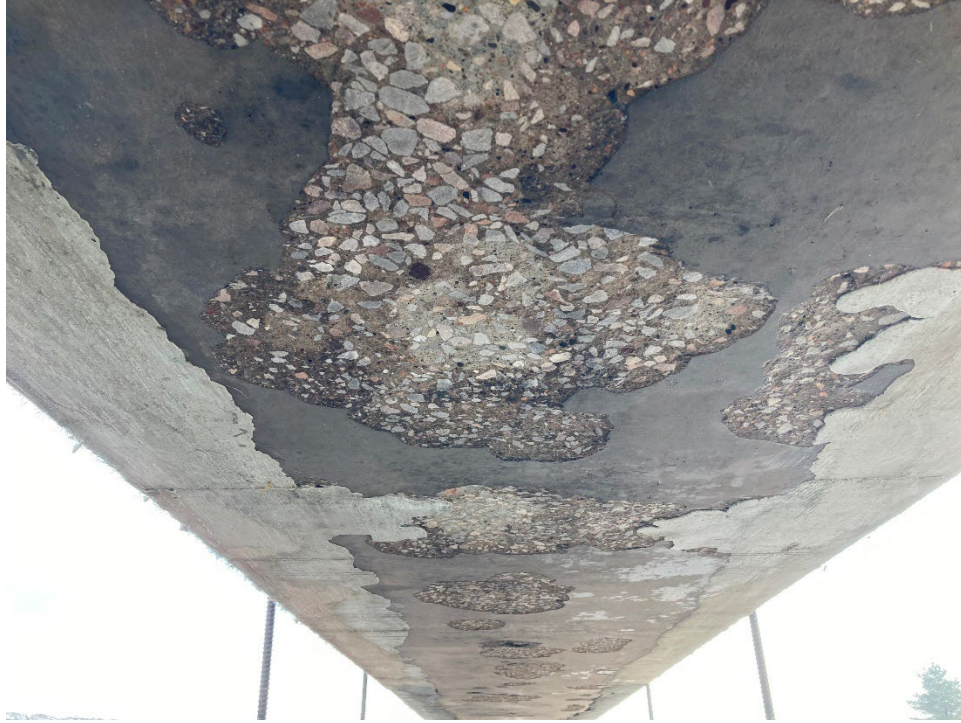
Figure 83. Bottom of girder spalls prior to repair
