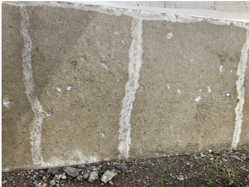
Figure 91. Closeup of vertical cracks in SCC/FRP repair section
