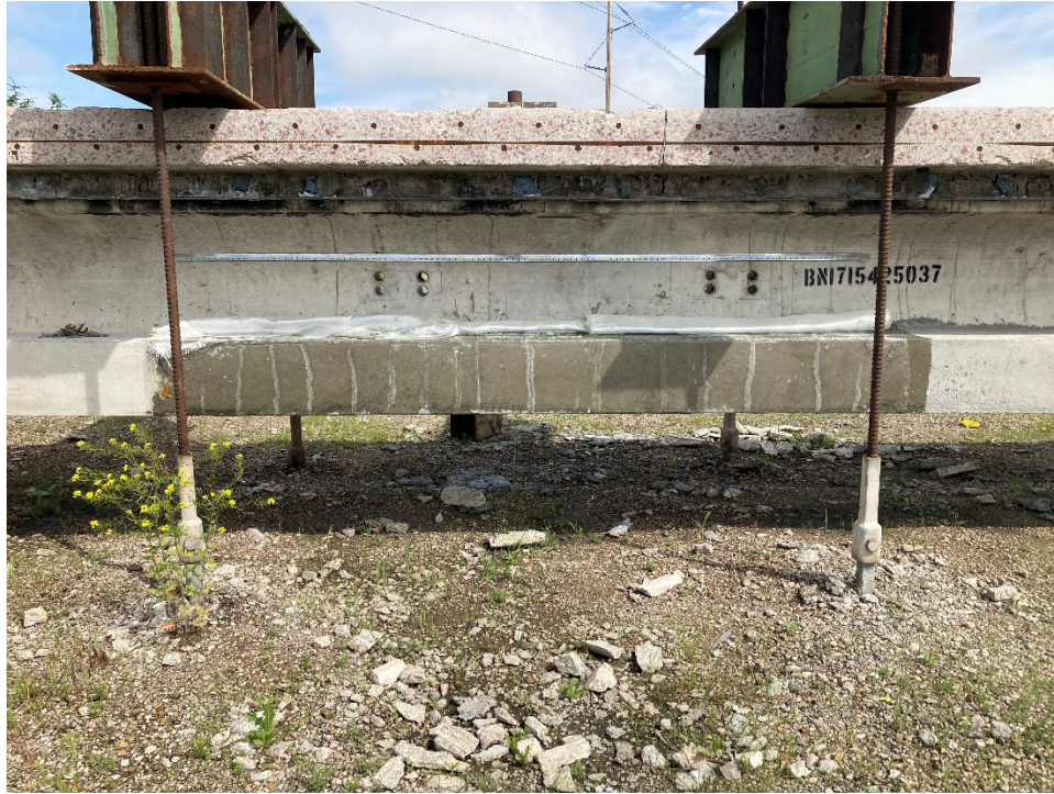
Figure 90. Vertical cracks in SCC/FRP repair section
