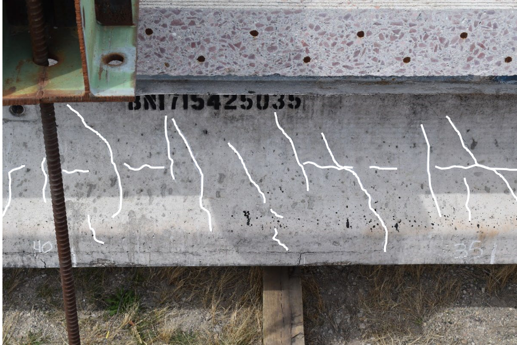
Figure 57. Cracking of Girder E bottom flange and web
