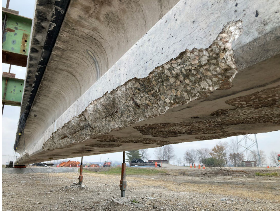
Figure 74. Bottom flange after loose concrete removal
