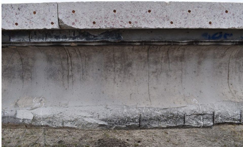
Figure 46. Bottom flange spalling on Girder E
