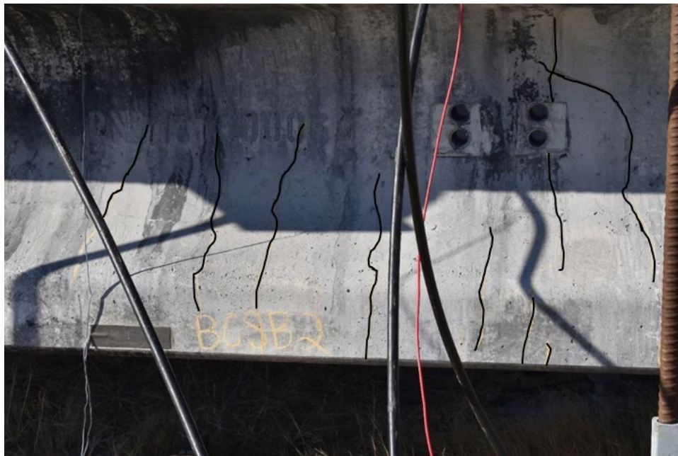
Figure 52. Crack patterns at midspan of Girder B
