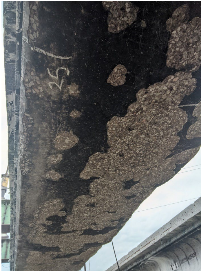
Figure 48. Bottom side spalling on Girder E
