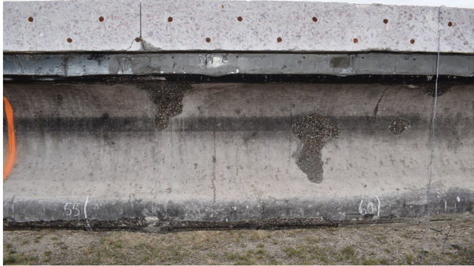
Figure 47. Web spalling on Girder E
