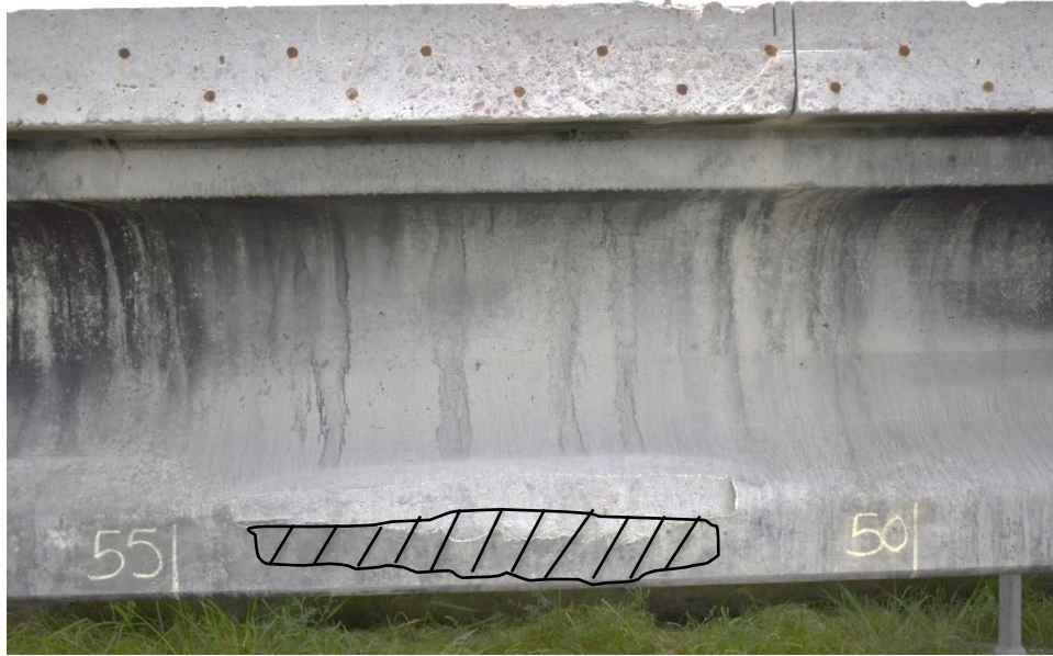
Figure 45. Spalled area on bottom flange near Girder B midspan
