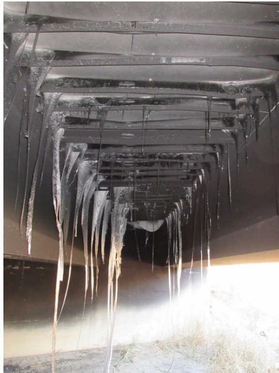
Figure 4. Melted polycarbonate stay-in-place forms
